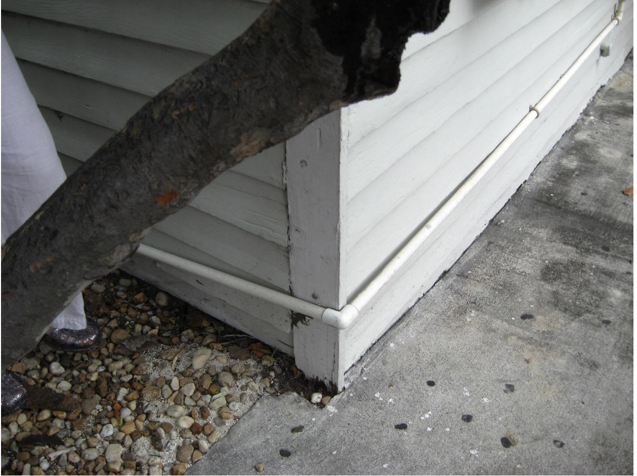
More wood rot and piping not supported
