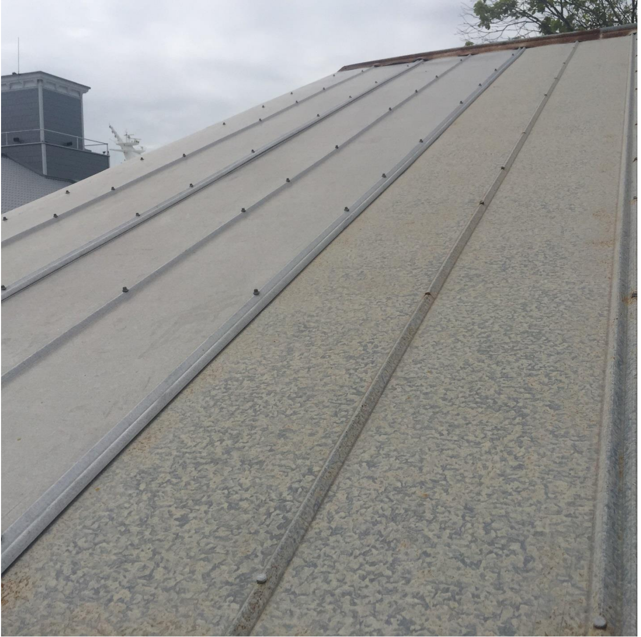
Old roofing needs replacing
