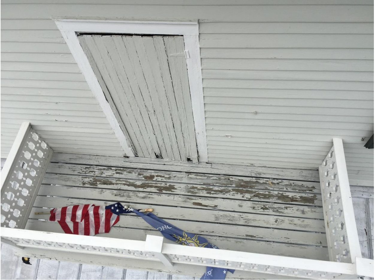
Porch loose and in need of repair
