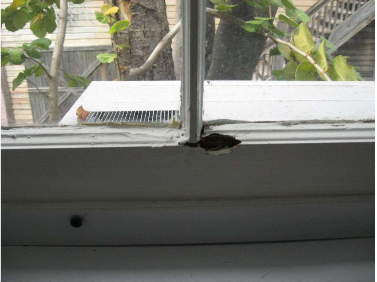
Window glazing bad and wood issues
