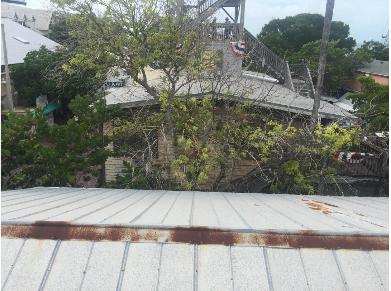
Roof damaged by trees
