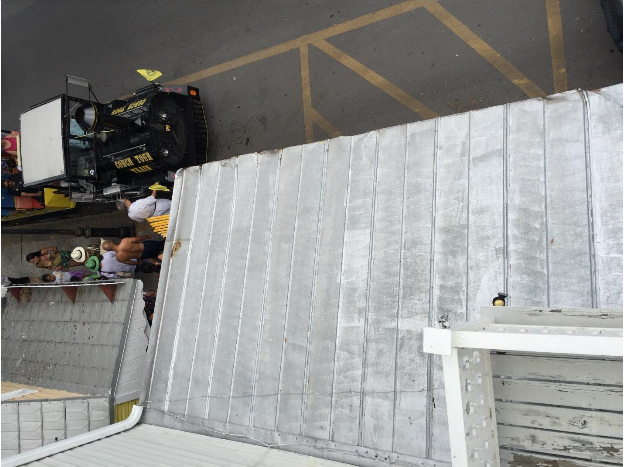
Lower roof damaged by trucks
