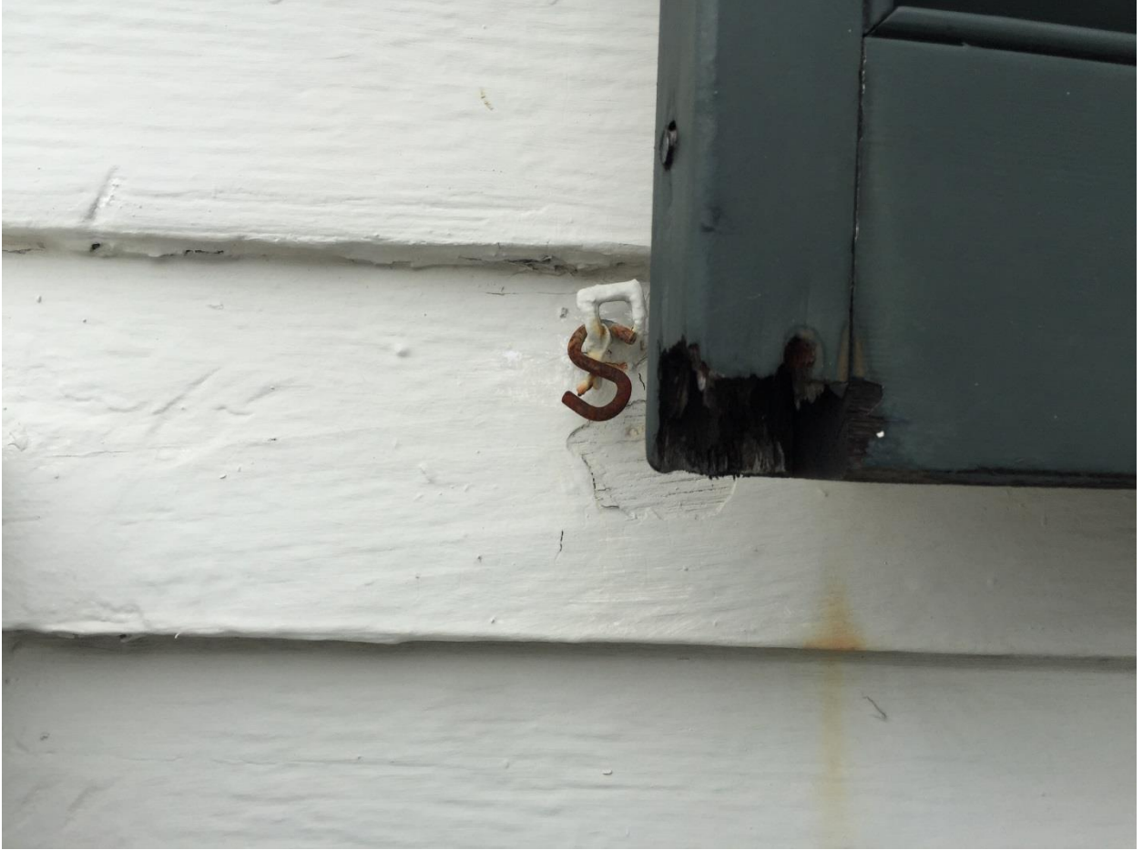
Shutter needs replacing
