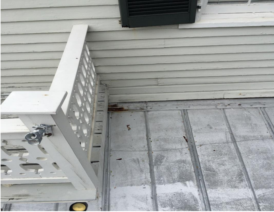
Flashing rusting. Needs repair
