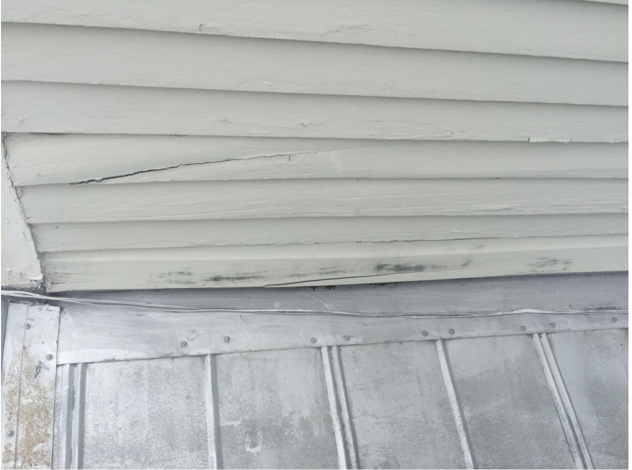
Second floor siding splitting and cable unsecured
