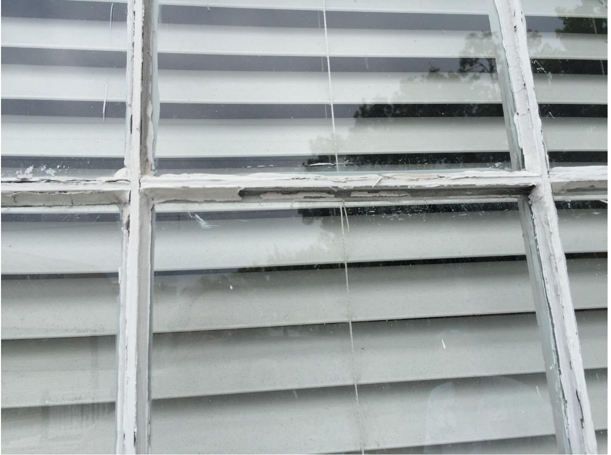
Outside window glazing bad
