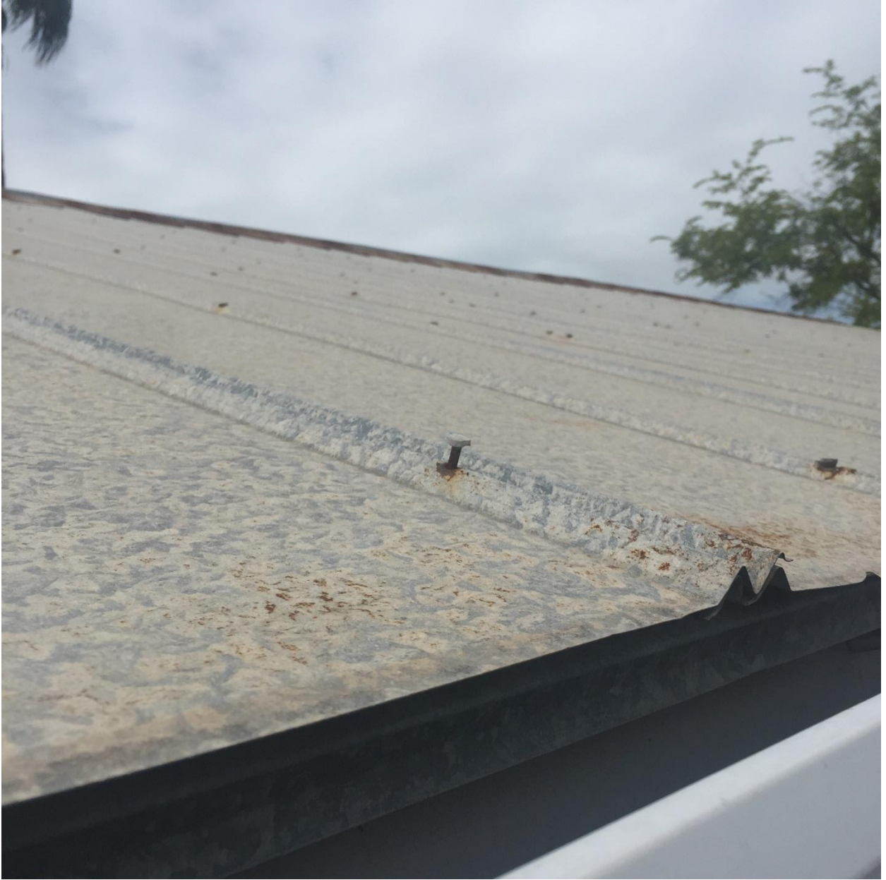
Roofing nails pulling loose
