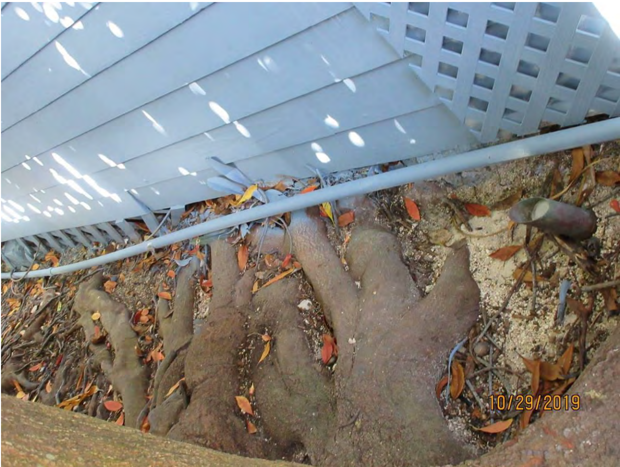
Photo of tree #1 showing roots in foundation area.
