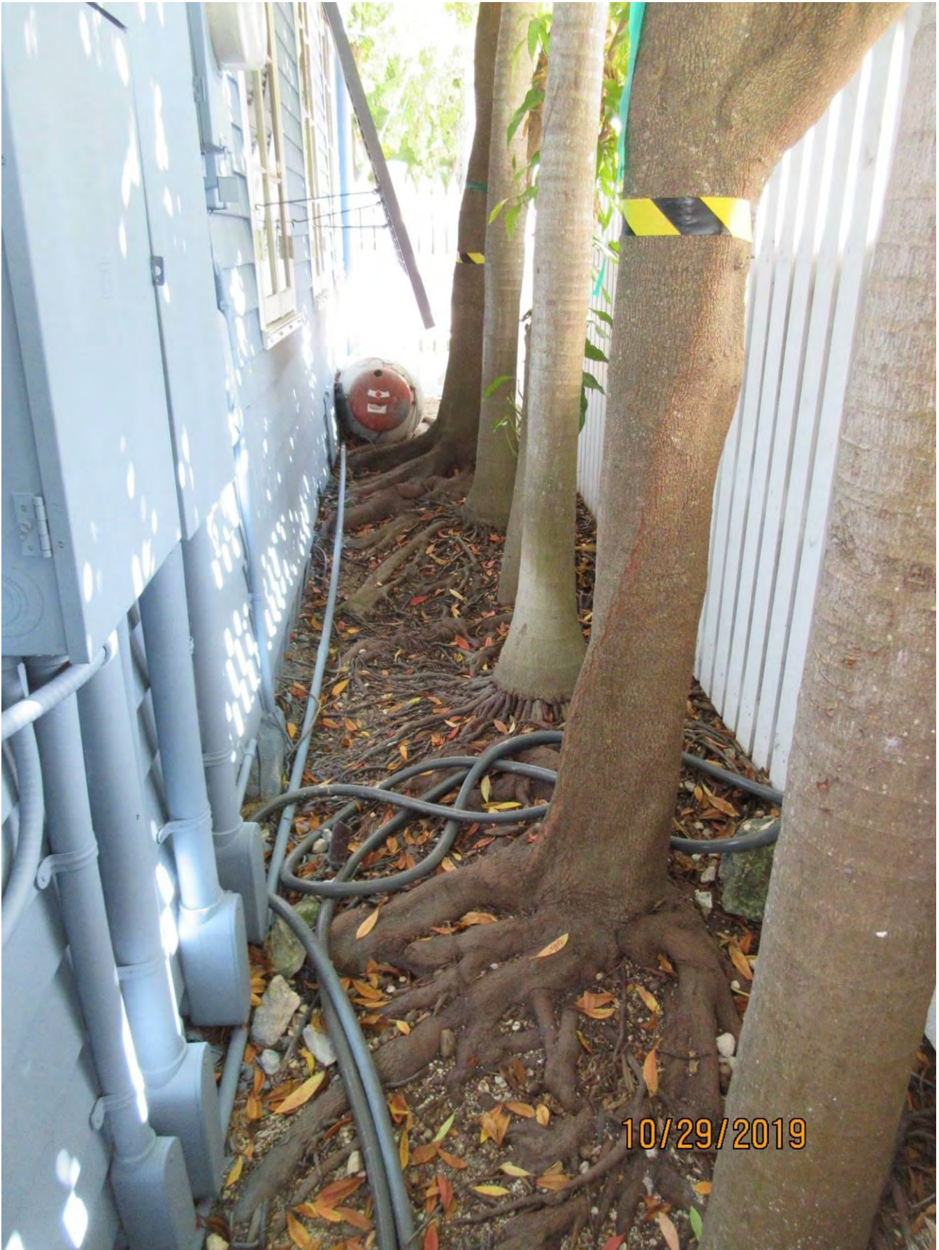
Photo showing root systems of trees 1-3 next to structure.
