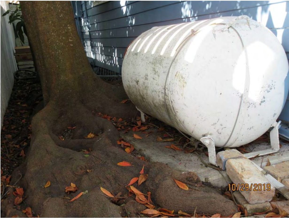
Photos of tree #1 showing roots impacting propane tank pad.
