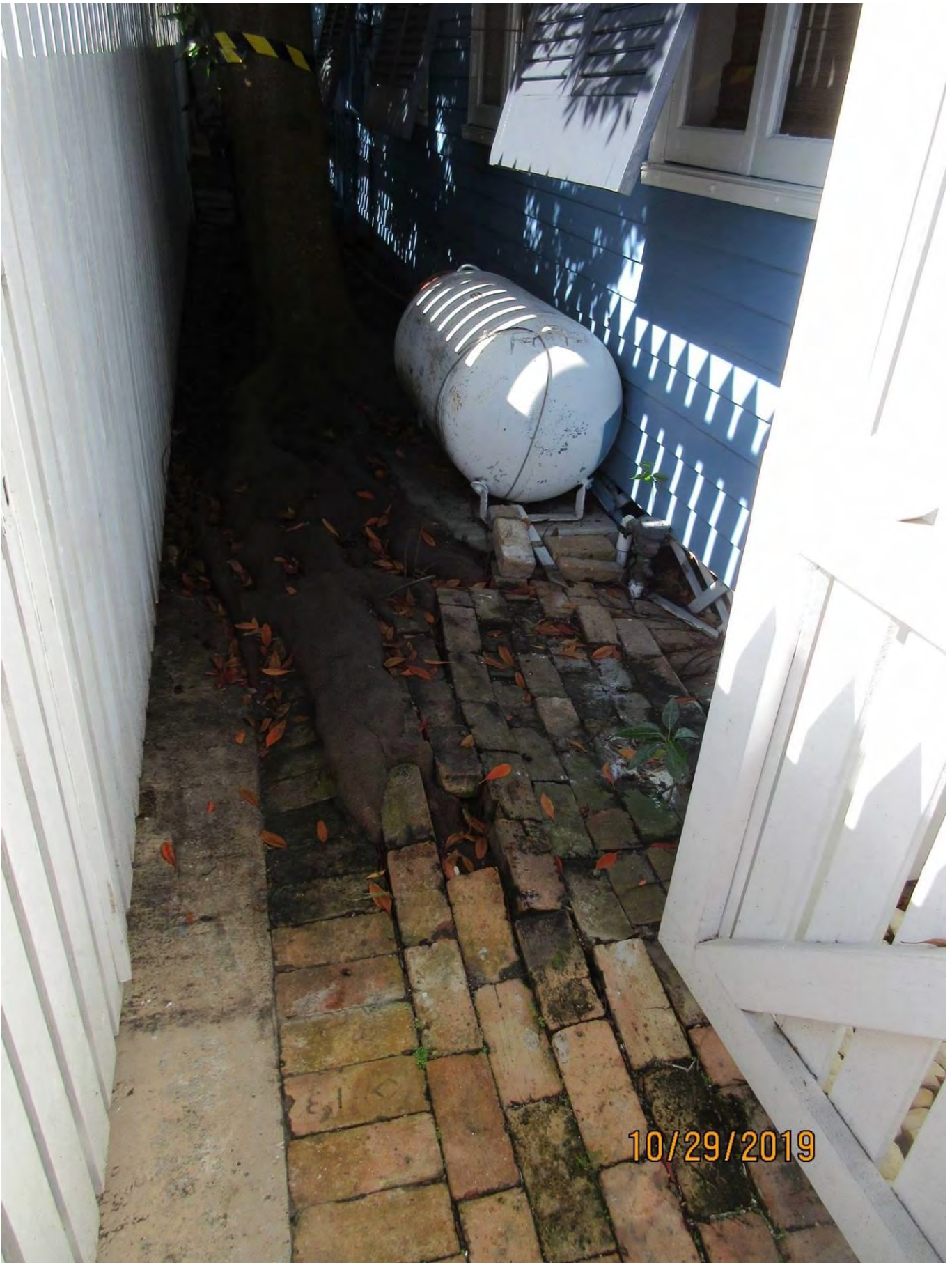
Photo showing the roots of tree #1, view 1.
