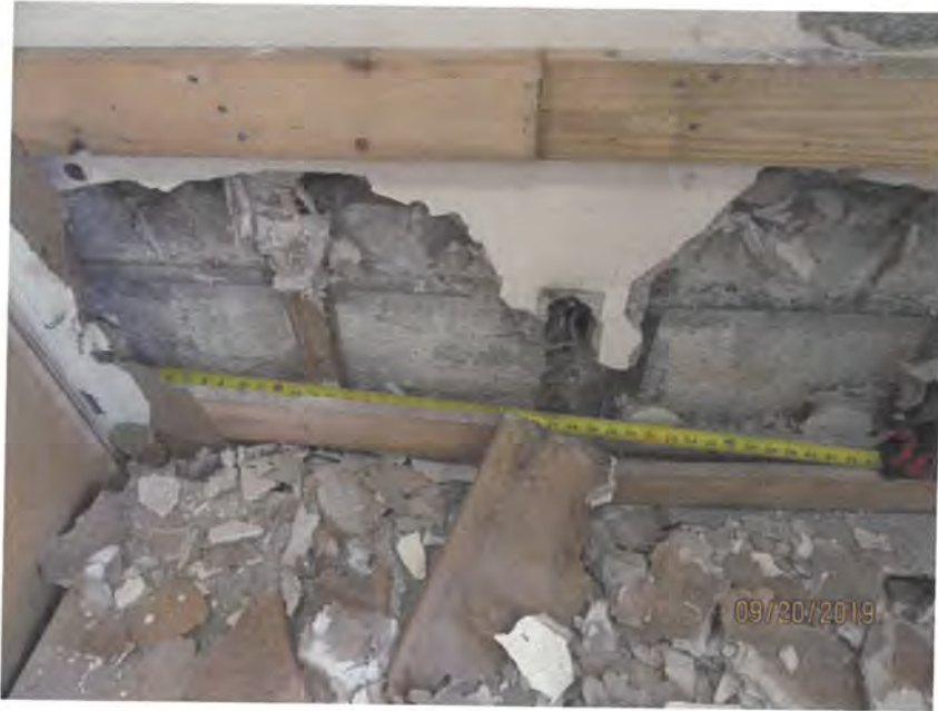
Cracked Foundation Stem Wall Opposite Mahogany
