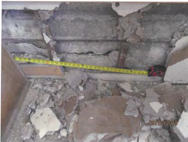
Cracked Foundation Stem Wall Opposite Royal Poinciana
