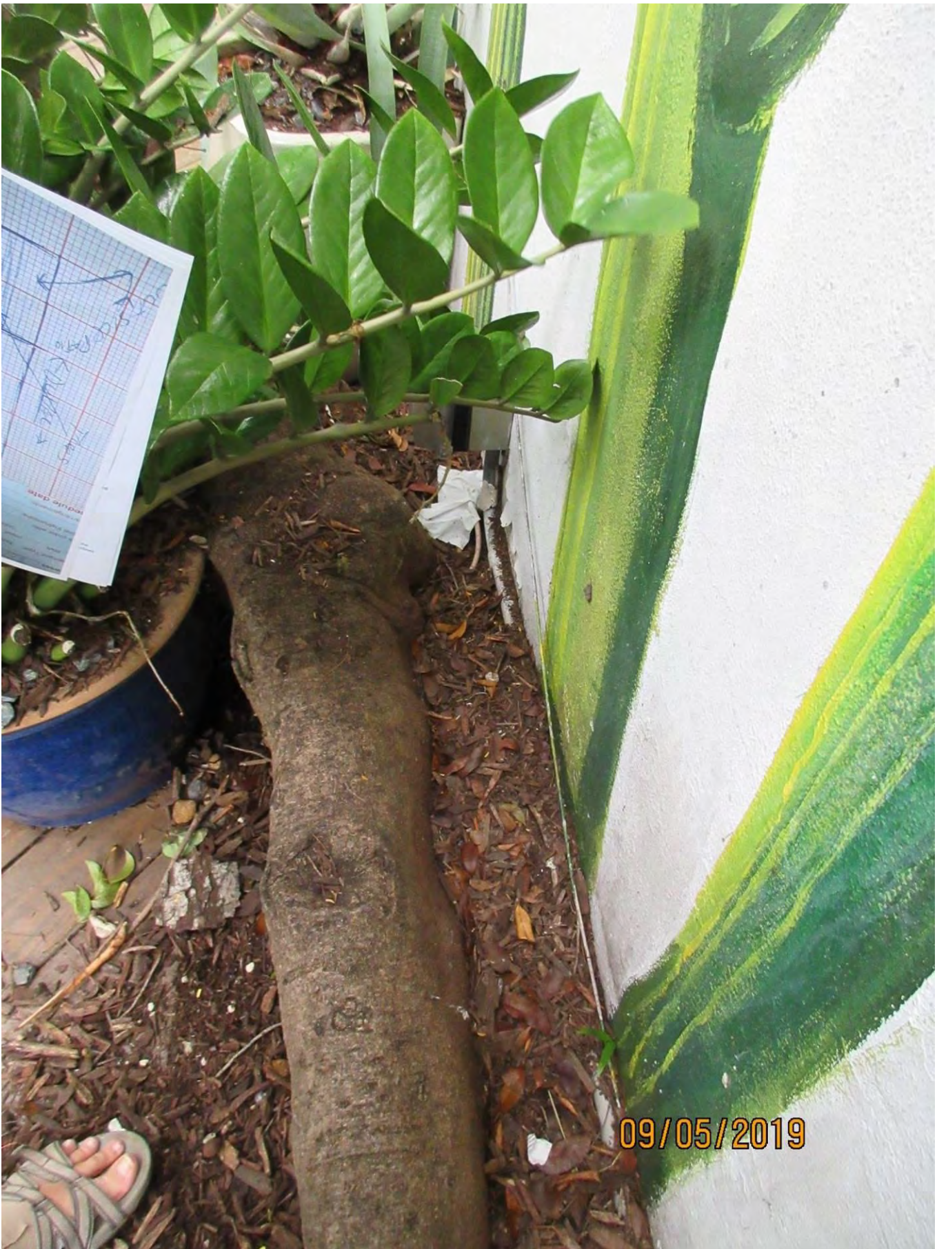
Photo showing base of Royal Poinciana tree against neighboring structure, view 2.
