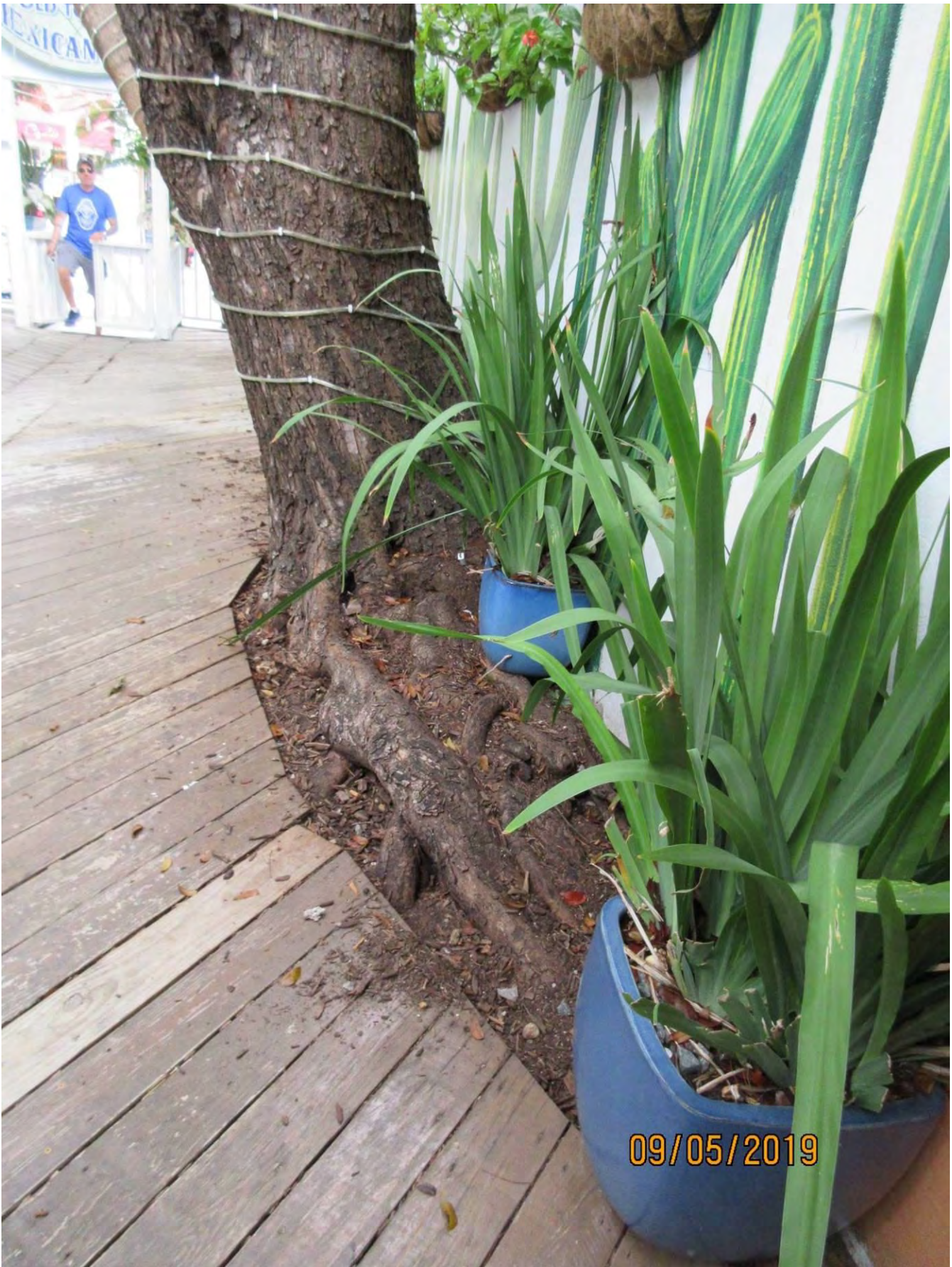
Photo of base of mahogany tree and tree roots against neighboring structure.
