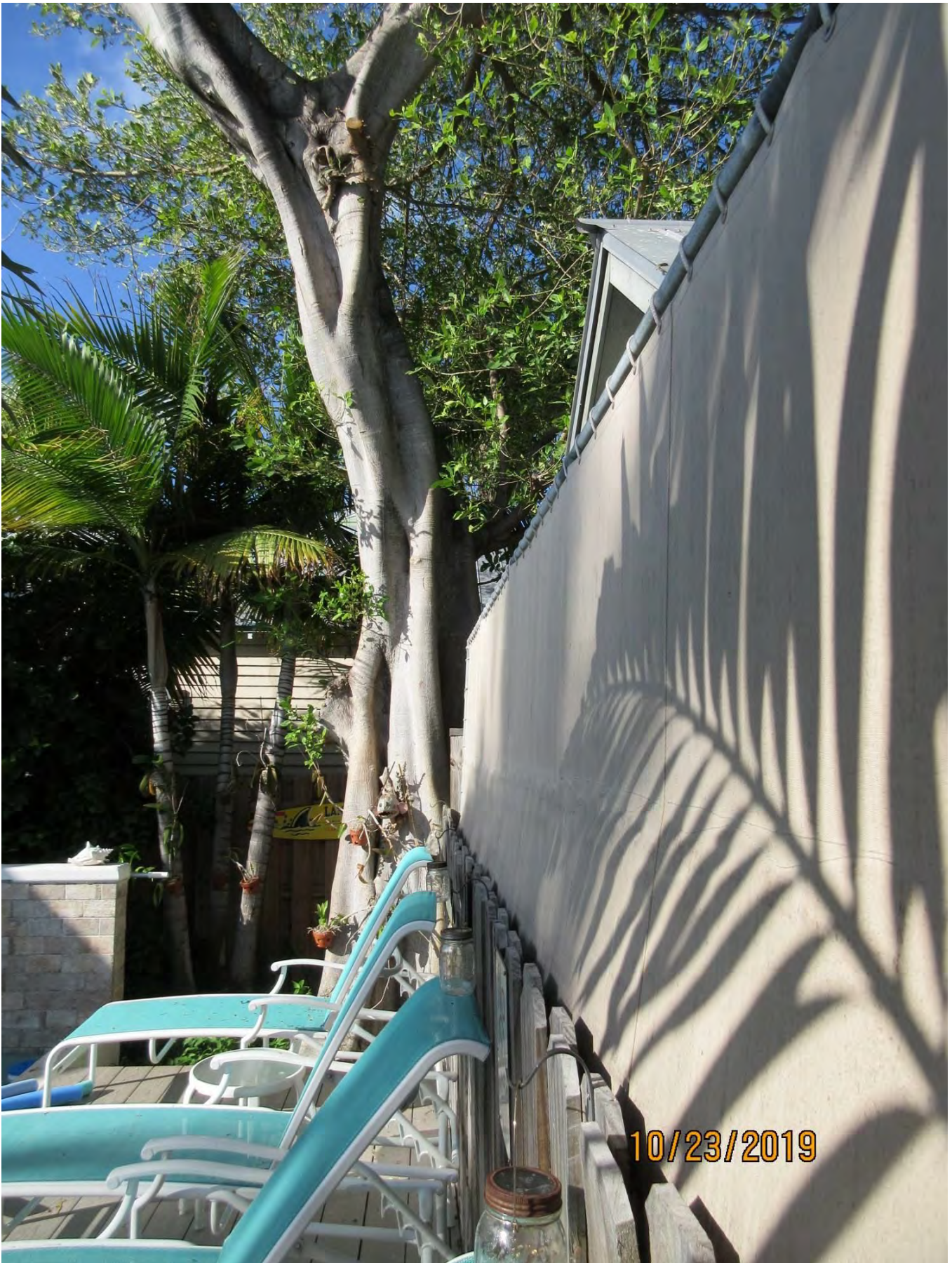
Photo showing tree trunk growing against fence, view 1.
