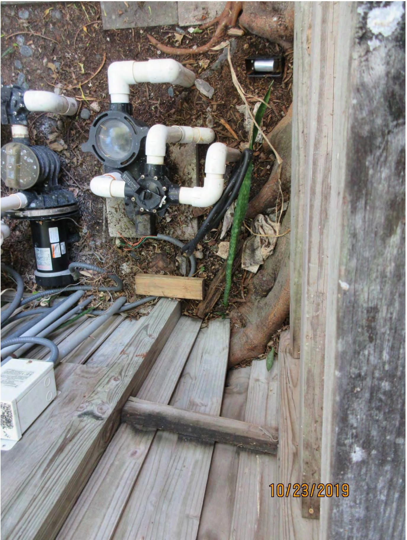
Photo looking over fence at neighbor's pump system, view 1.
