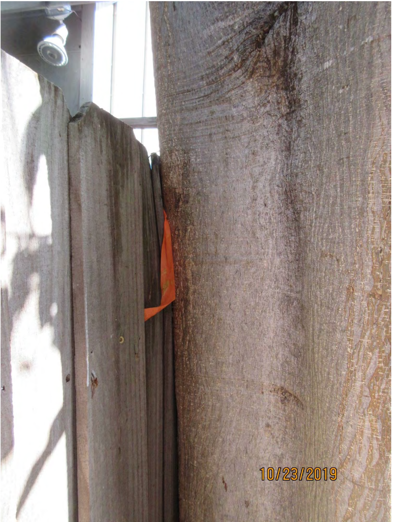
Photo showing tree trunk growing against fence, view 2.
