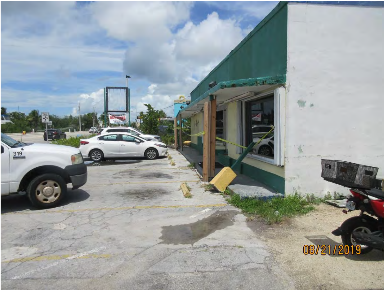
Photo of property looking toward the east across the front of the existing structure.
