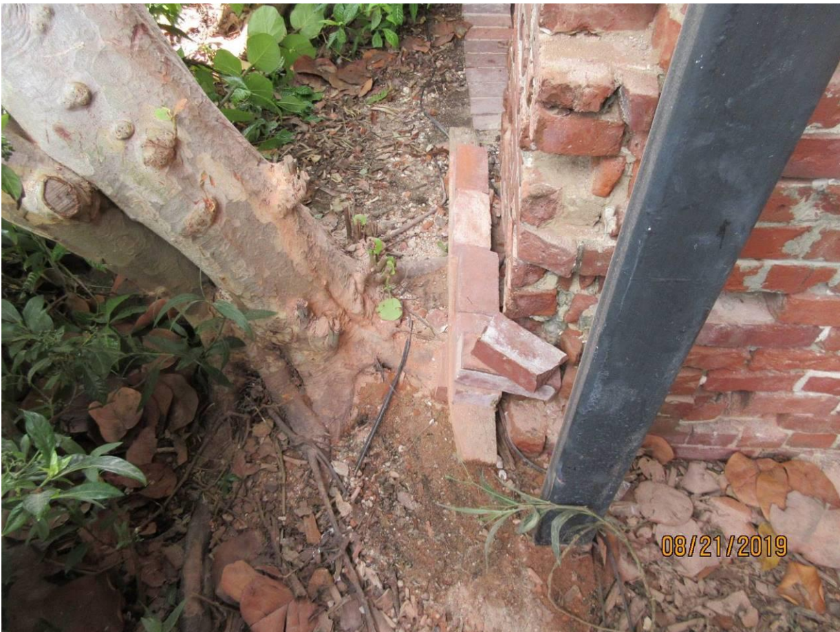
Photo showing base of tree close to wall, view 1
