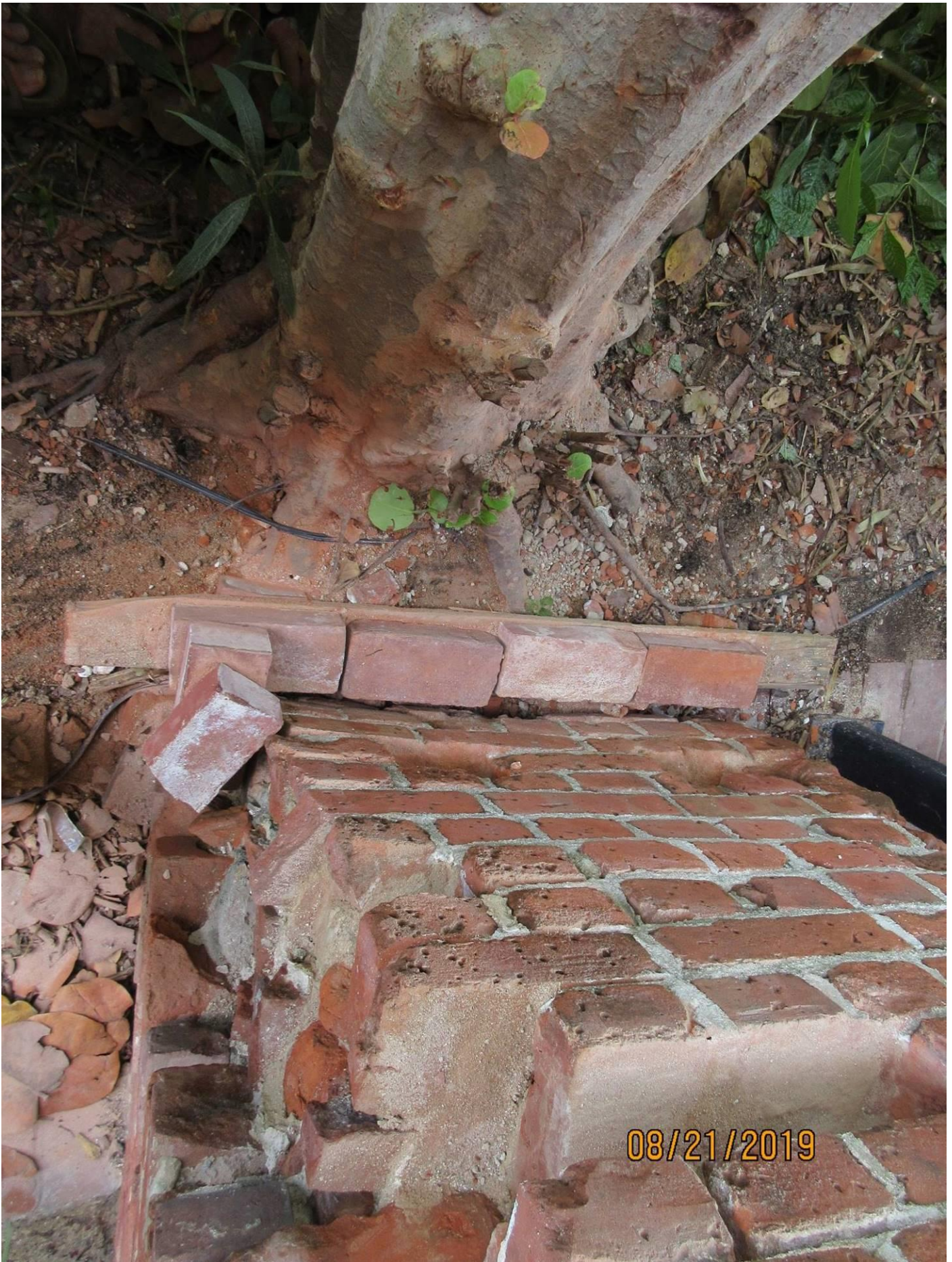
Photo showing base of tree close to wall, view 2.
