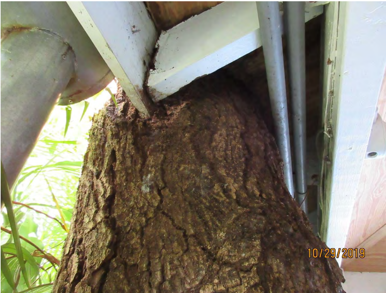
Two photos showing roof of structure against and partially imbedded in tree trunk.
