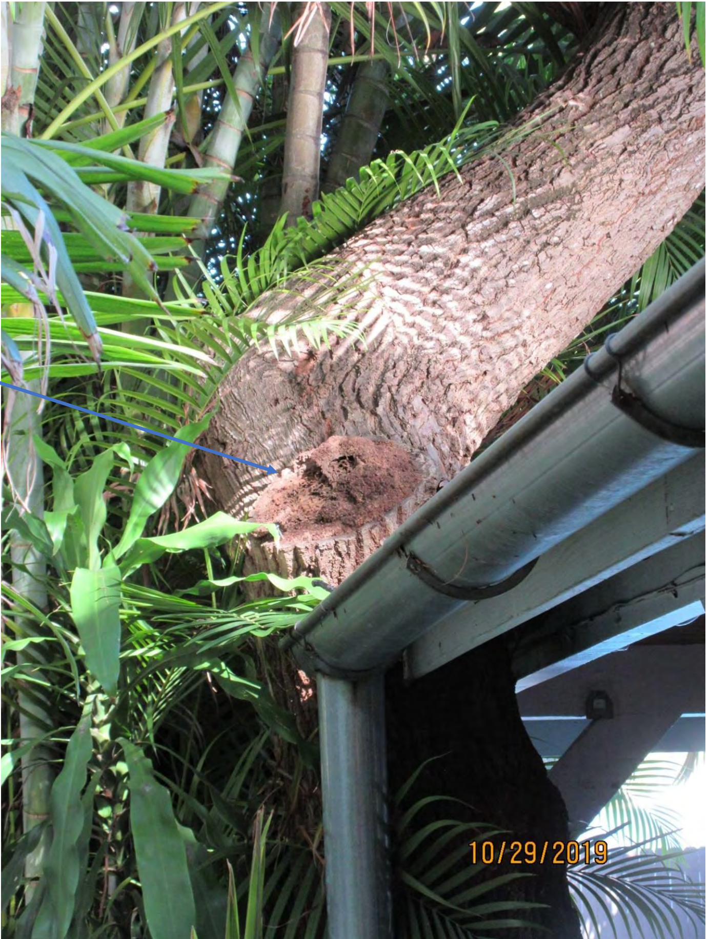
Photo of trunk of tree. Note evidence of termite frass in old cut.
