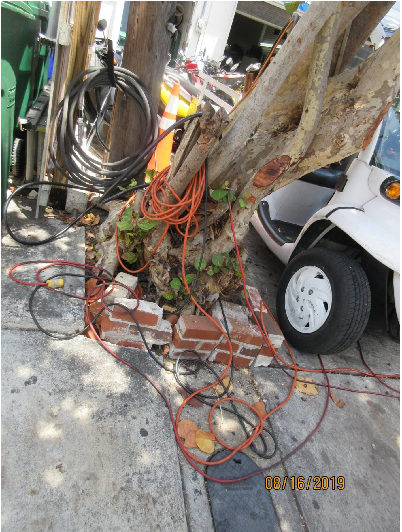
Photo of base of tree showing water meter location and utility pole view 1.
