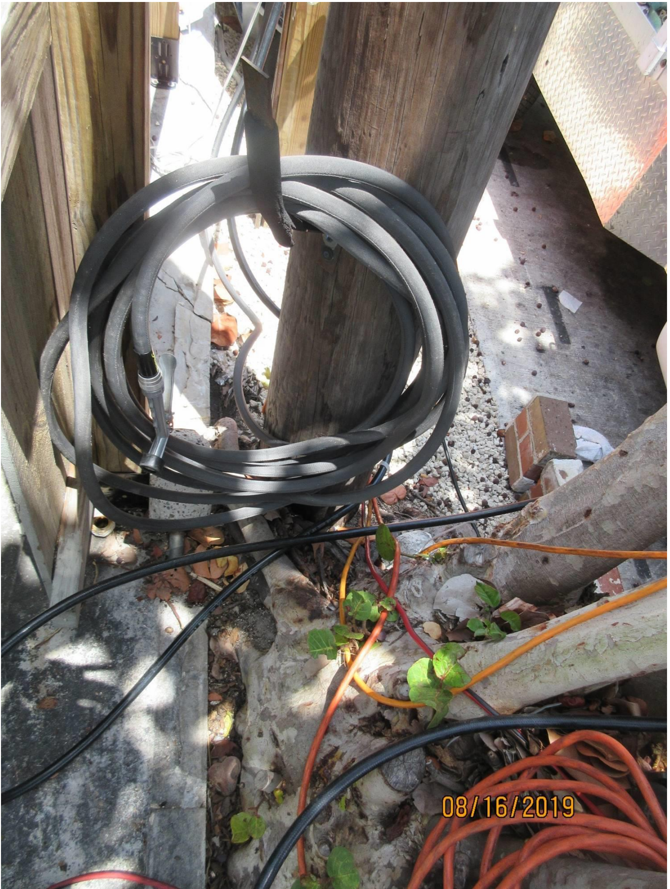
Photo of base of tree showing utility pole location.
