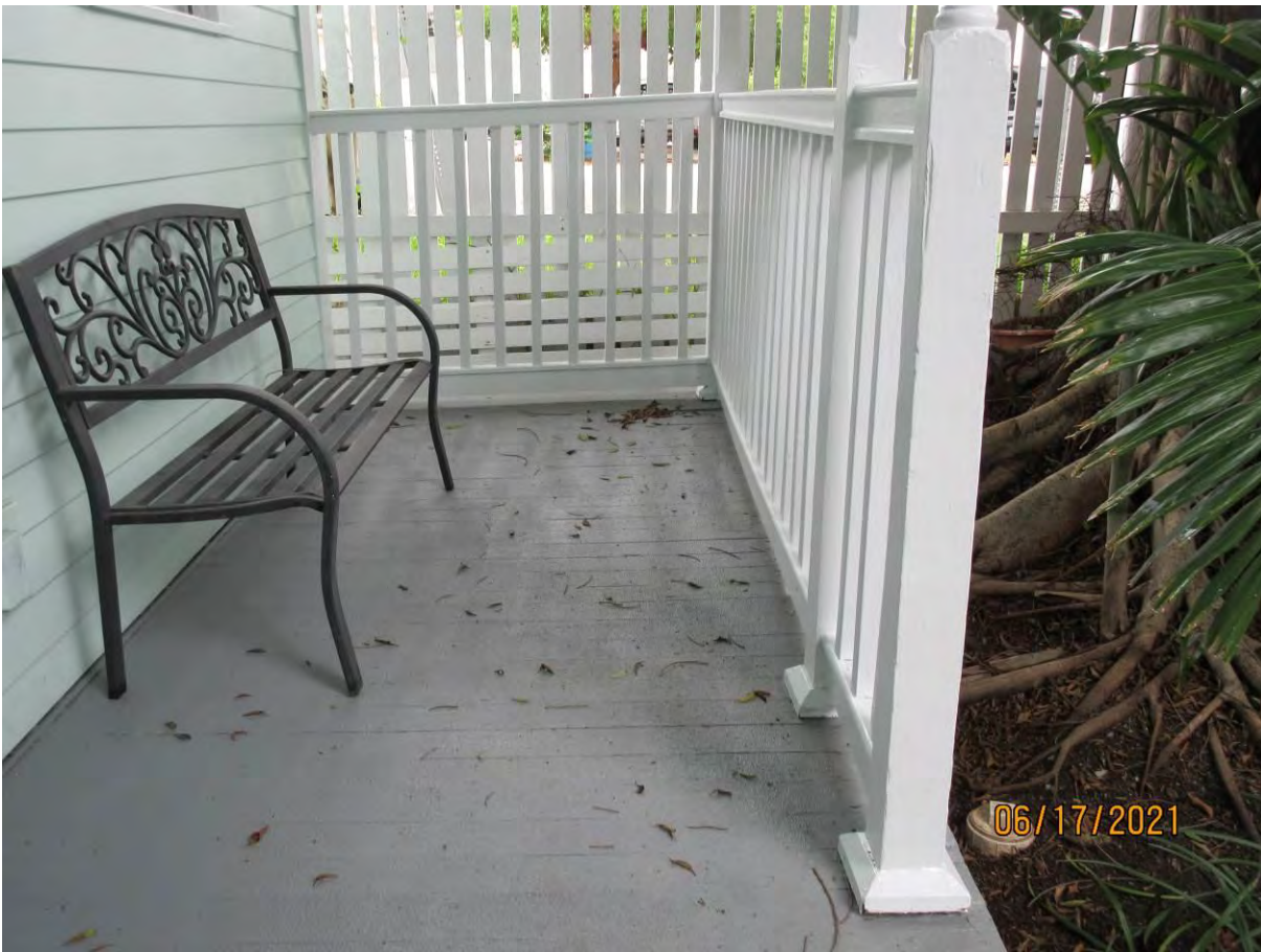
Photo showing porch area. Top right corner is uplifted.
