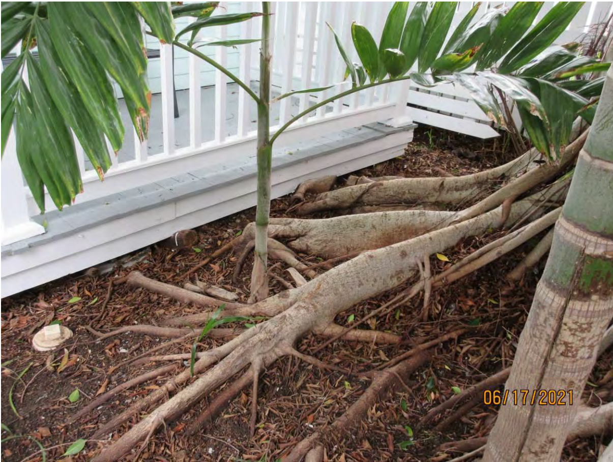
Photo showing tree roots in relation to structure.
