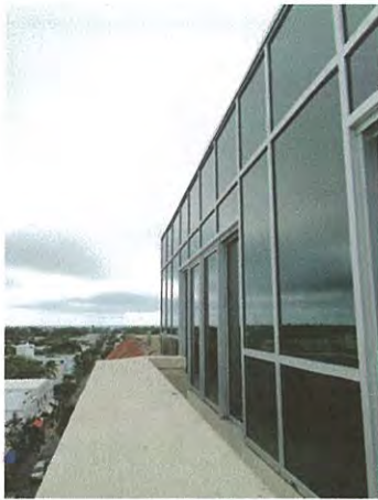
EXTERIOR CURTAIN WALL
