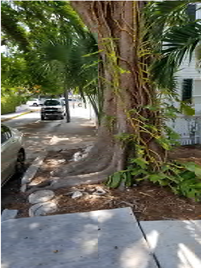
Photo 2. View of tree from north. Sidewalk is missing, adjacent pavers and curb broken.
