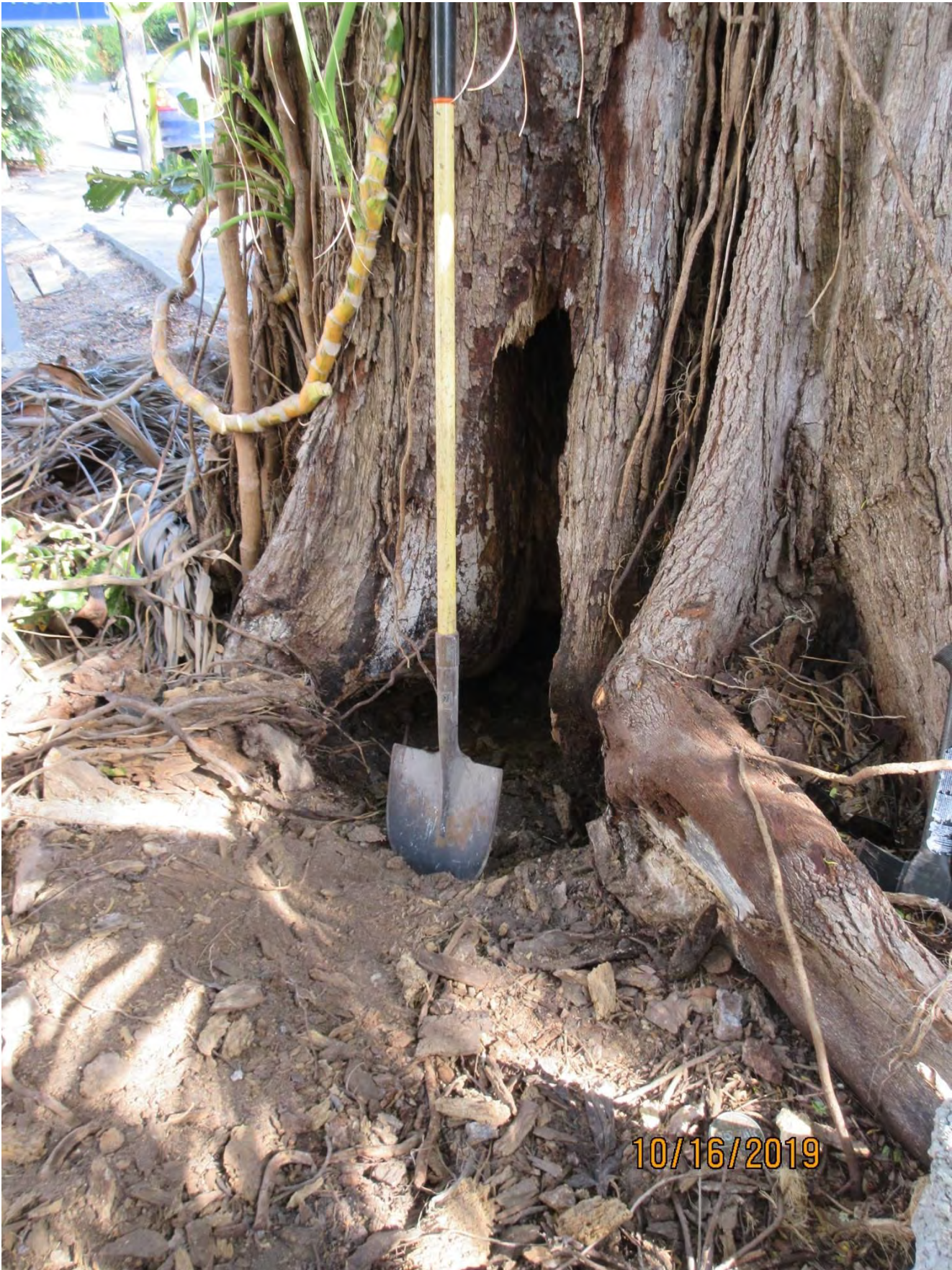
Photo showing base of tree hole area with a shovel to show size of area.
