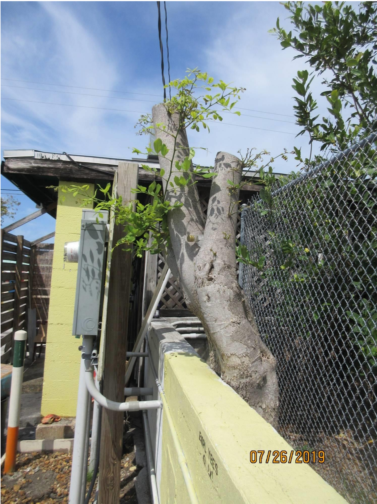
Photo of tree #1, Jamaican Dogwood. Note location of electrical lines and conduit
