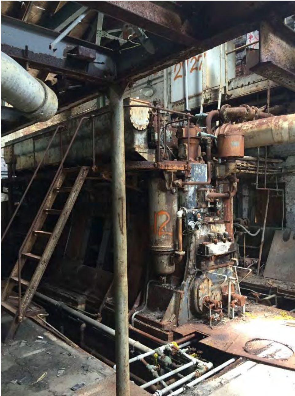
PHOTO 2: Inactive generator inside buildings at the Site
