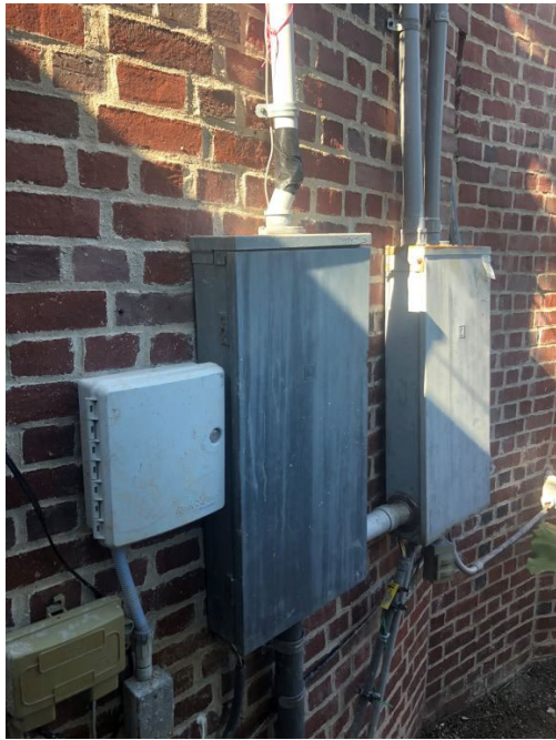
Main Electrical Panel to be replaced
