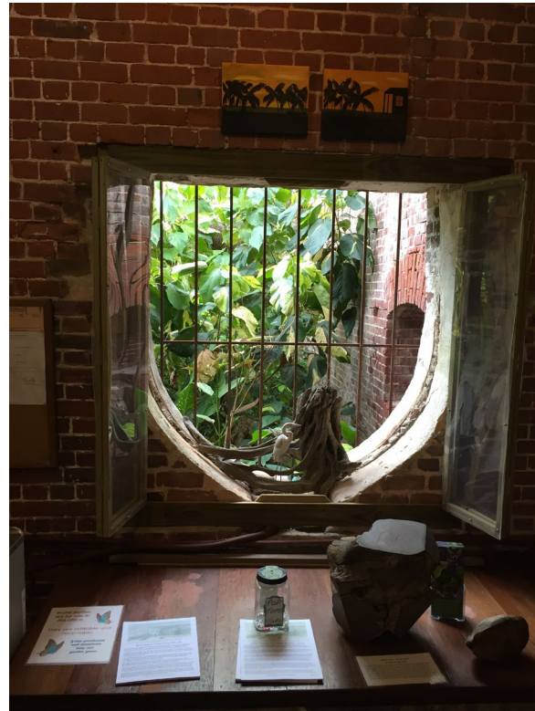
Meeting Room Window to be Replaced
