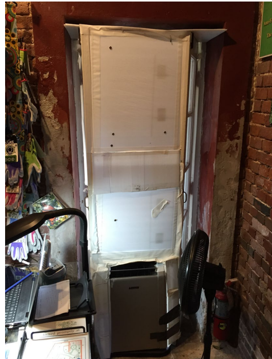
3' Side Door to be Replaced
