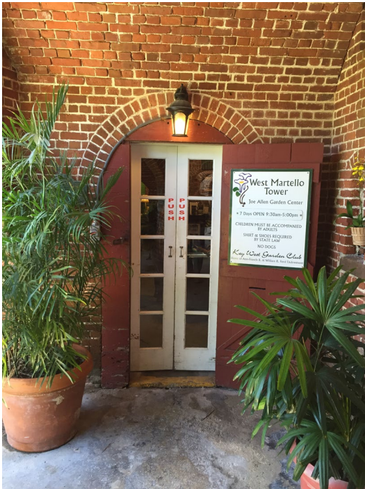
3' Entrance Door to be Replaced
