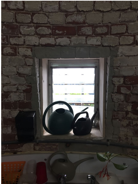
Break Room Window to be Replaced
