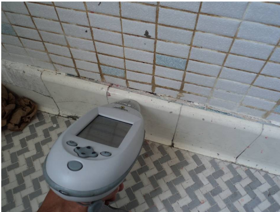
Photograph #12: Lead identified on ceramic baseboard (XRF # 272).
