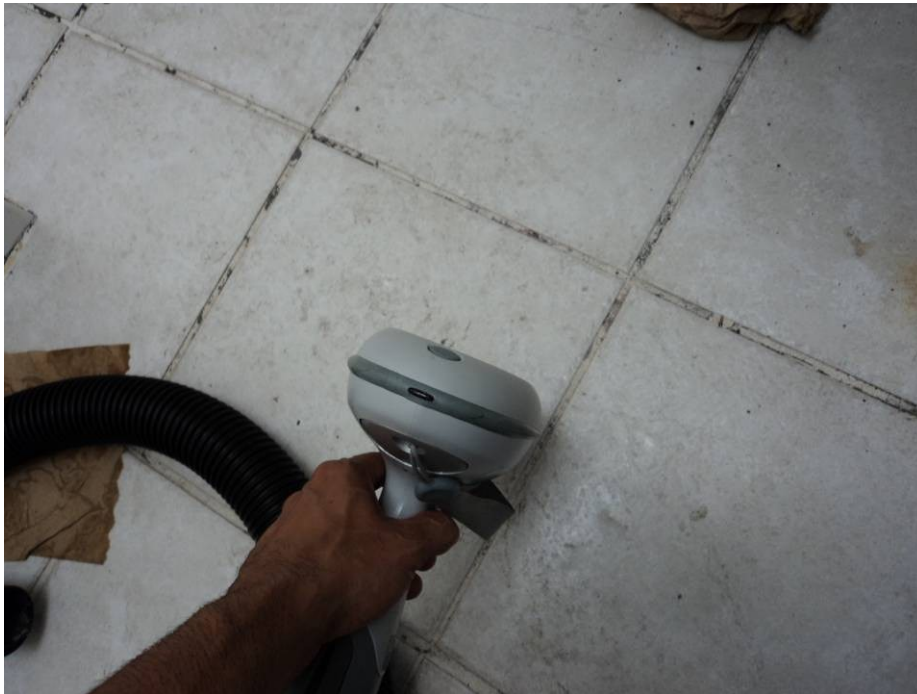
Photograph #7: Ceramic tile identified with lead during this inspection (XRF#212).
