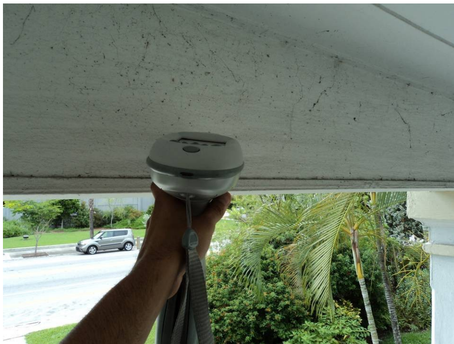
Photograph #24: Exterior wood beam paint identified with LBP during this inspection (XRF #548).
