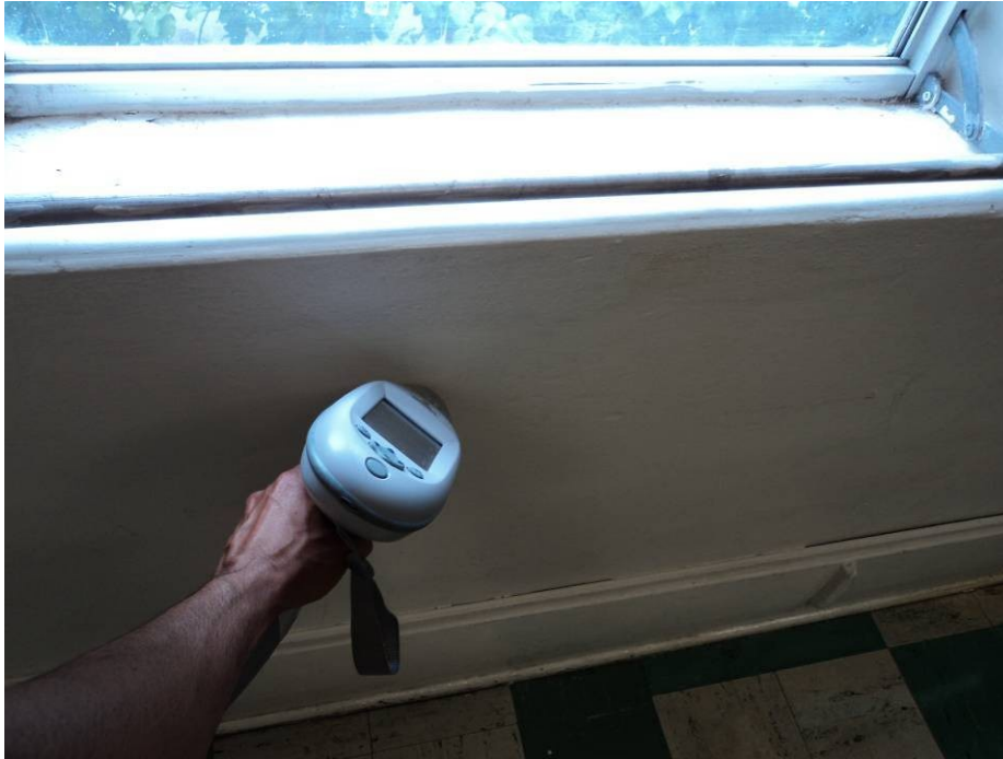
Photograph #13: LBP identified on wall during this inspection (XRF #287-288).
