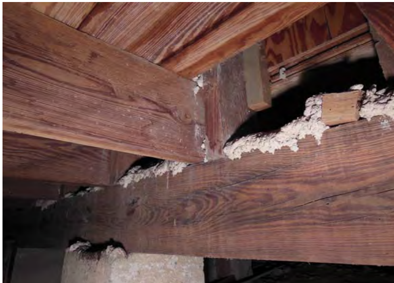
#7 Auditorium First Framing Existing Condition: Wood Joist / Tongue-and-Groove Plank on Wood Girder
