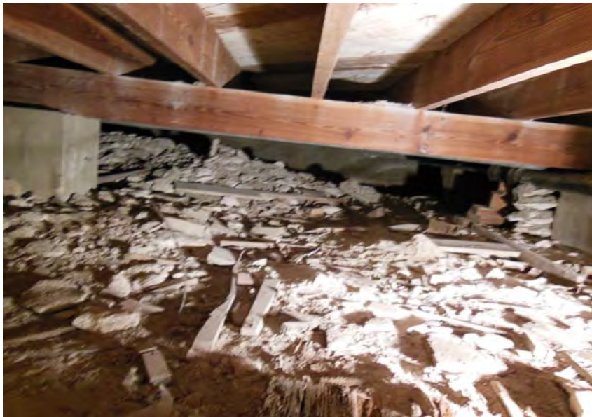
#3 Building A Foundation Existing Condition: Ground Floor Framing and Interior Spread Footing
