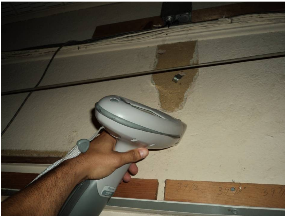
Photograph #6: Wall paint identified with LBP (XRF #113).
