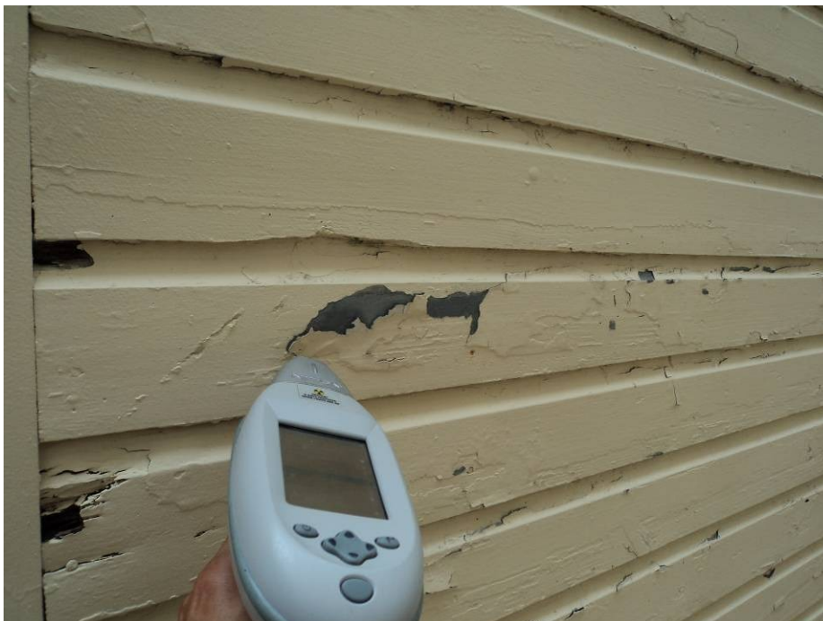
Photograph #20: LBP in poor condition identified on exterior wood shed attached to the Auditorium building (XRF #512)
