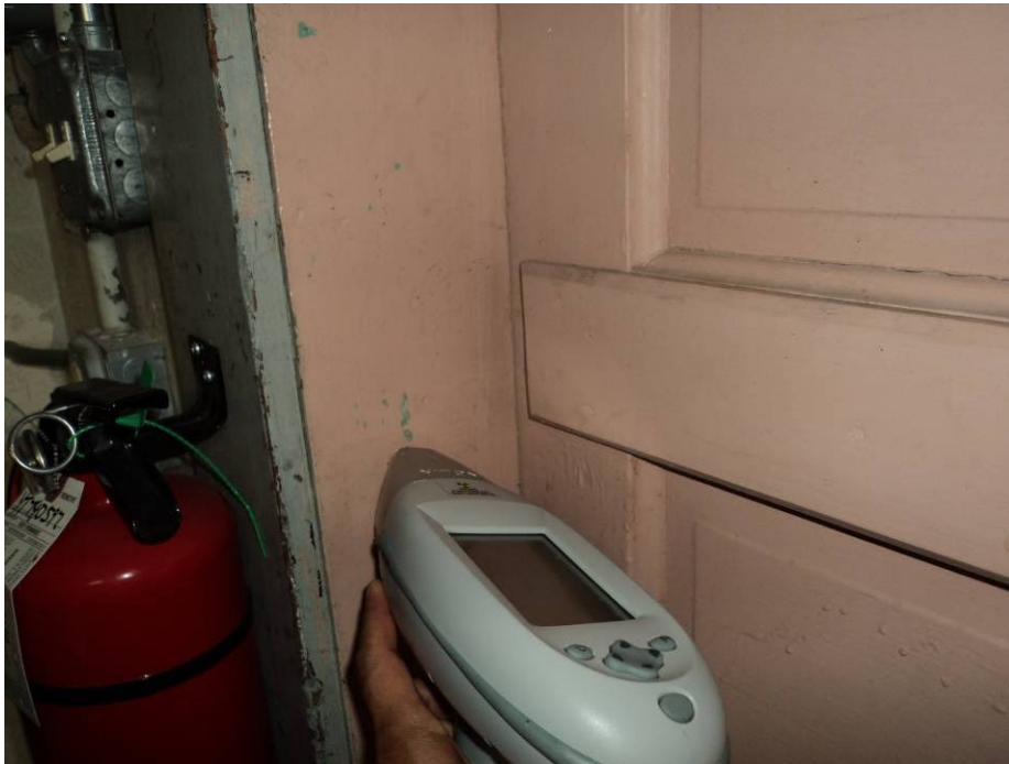
Photograph #9: Door and door casing identified with LBP during this inspection (XRF #182-183).
