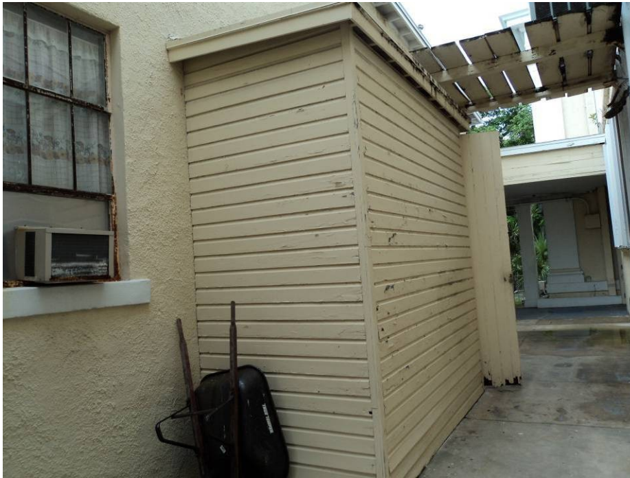
Photograph #19: LBP in poor condition identified on exterior wood shed attached to the Auditorium building (XRF #512)
