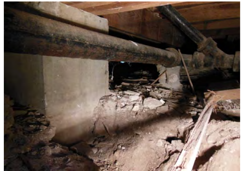
#4 Building B Foundation Existing Condition: Ground Floor Framing and Interior Spread Footing
