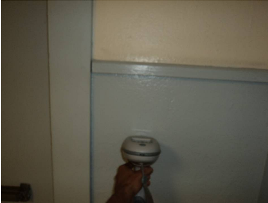
Photograph #5: Wall paint identified with LBP (XRF #39).
