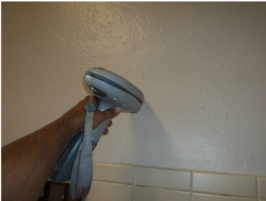
Photograph #2: Wall paint identified with LBP (XRF #25).
