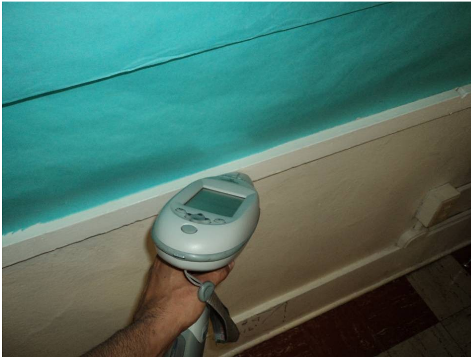
Photograph #11: LBP identified on wood trim during this inspection (XRF #256-257).
