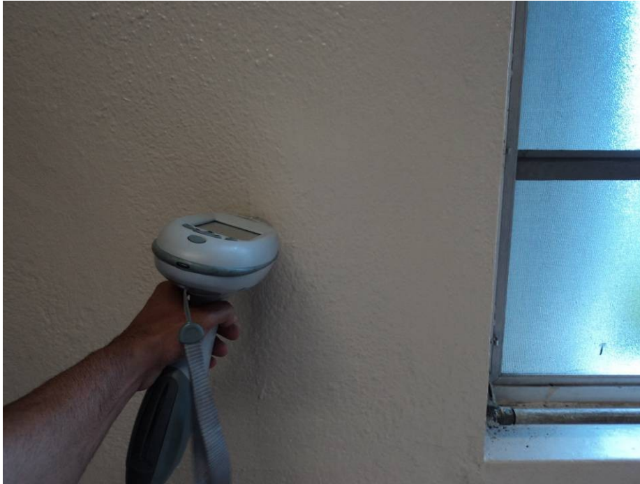
Photograph #3: Wall paint identified with LBP (XRF #28).
