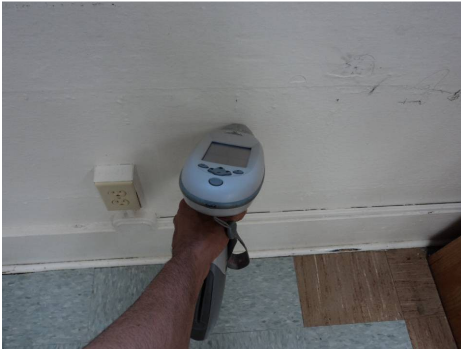
Photograph #15: LBP identified on classroom wall (XRF #368).
