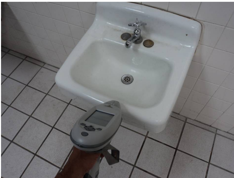
Photograph #16: Lead identified on metal sink.
