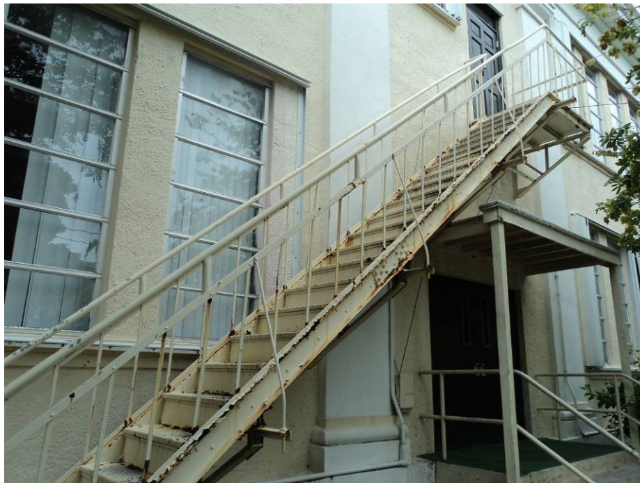
Photograph #22: Typical exterior stairwell identified with LBP during this inspection.
