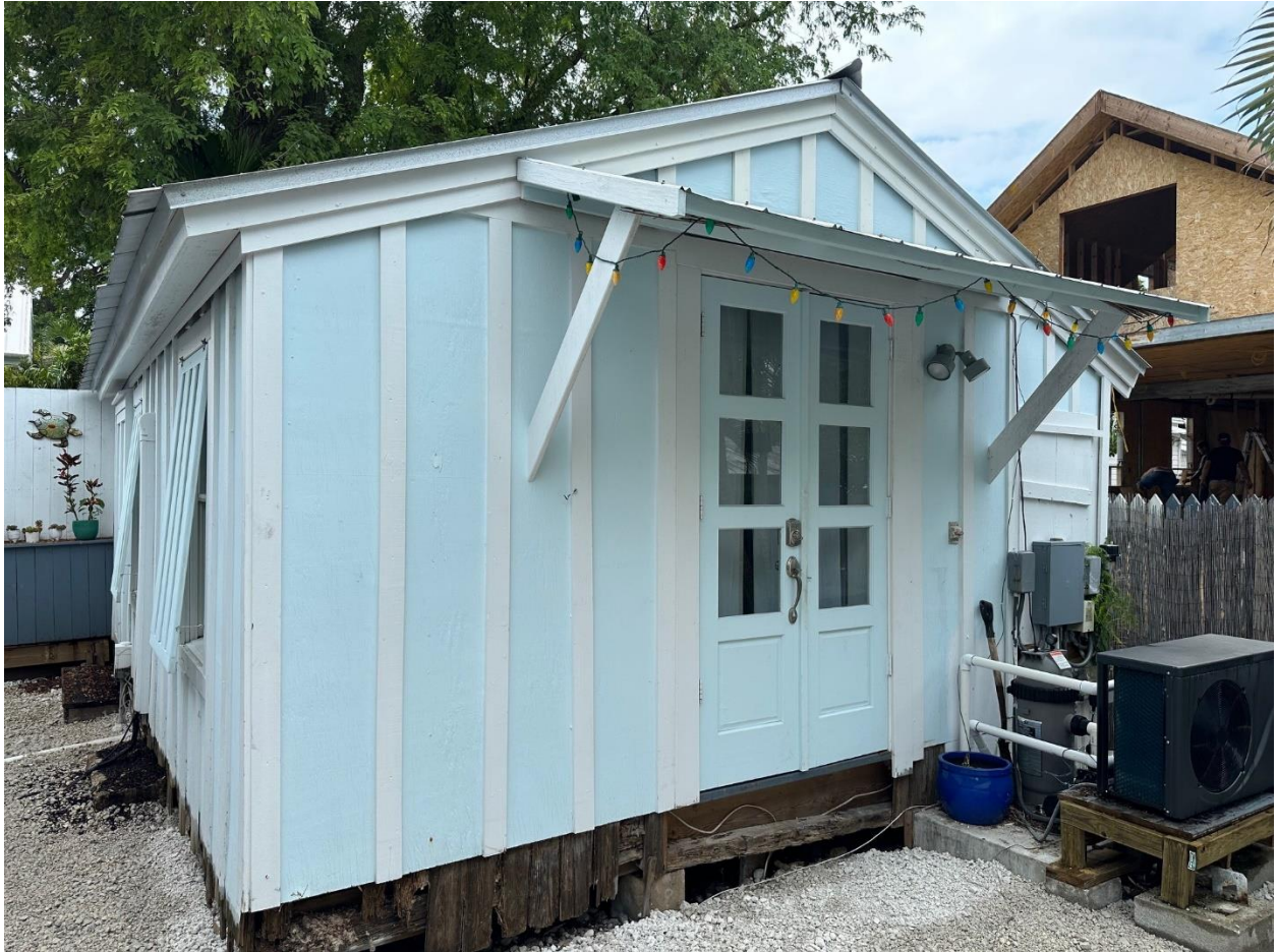
Current accessory structure. Notice deteriorated floor beam and siding at bottom.
