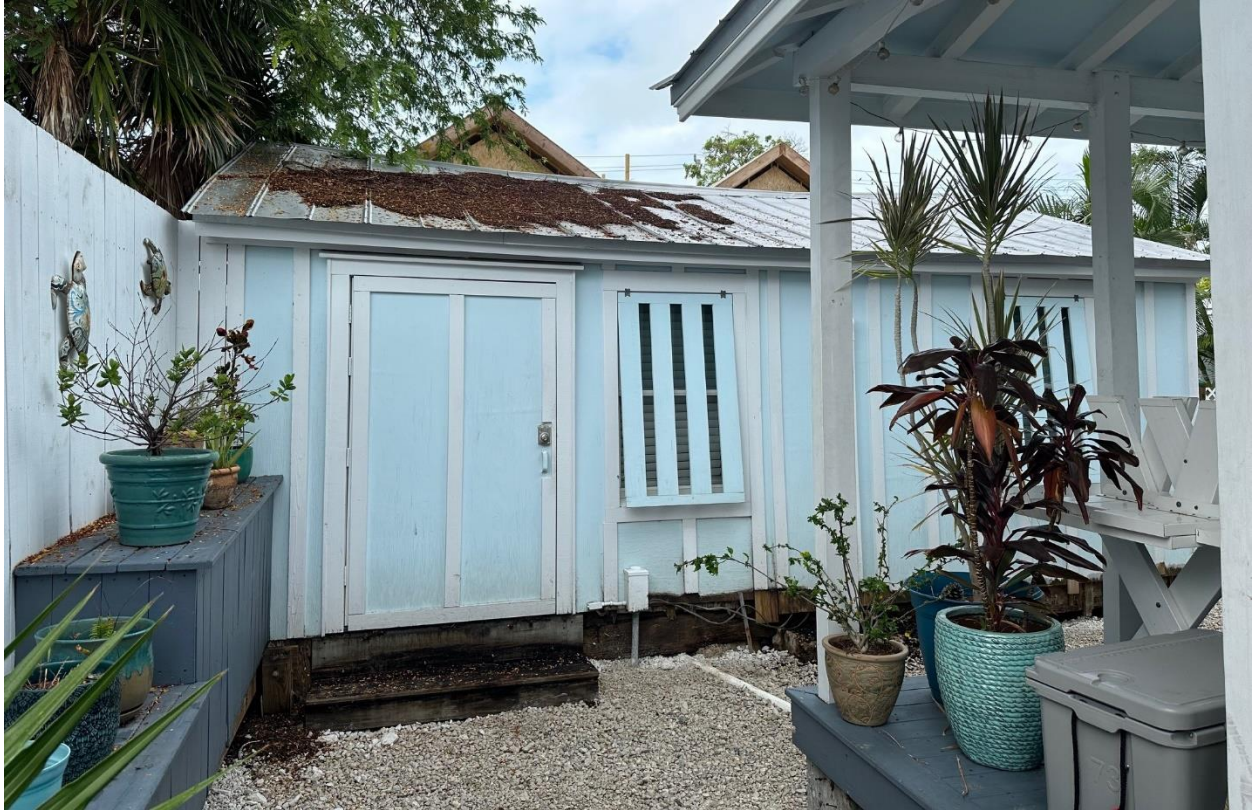
Current accessory structure. Notice deteriorated floor beam and siding at bottom.
