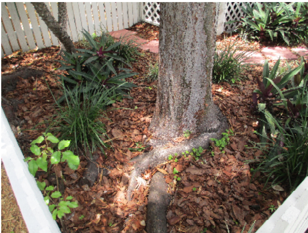
Roots effecting fence and pathway pavers
