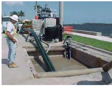
Pit w/ bentonite drilling mix. 10" HDPE FM being pulled through bore hole.
