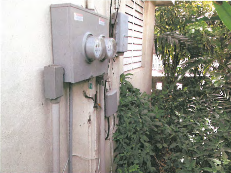
Equipment (Electrical Panel)
