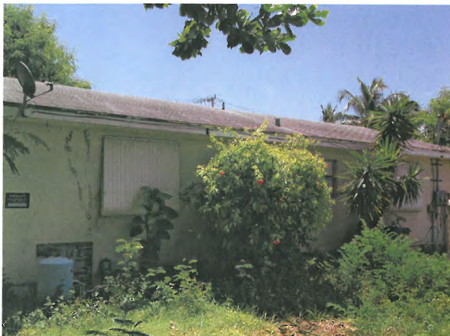
Rear View & Electrical Panel 8/21/12
