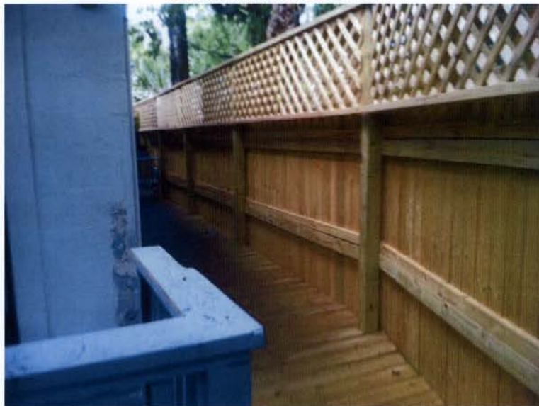
SOUTH WEST SIDE OF HOUSE LOOKING TOWARDS THE FRONT RED TAGGED DECK & FENCE
