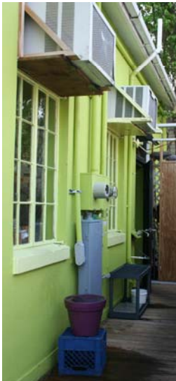
Water collection from A/c Units to water plants
