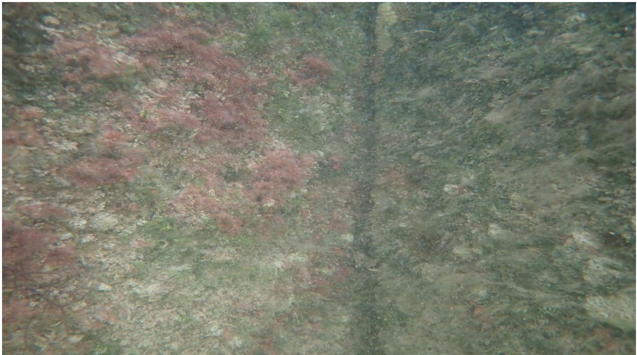
Photo 8. Jetty at the terminus of Duval Street with concrete seawall face showing attached filamentous algae.
