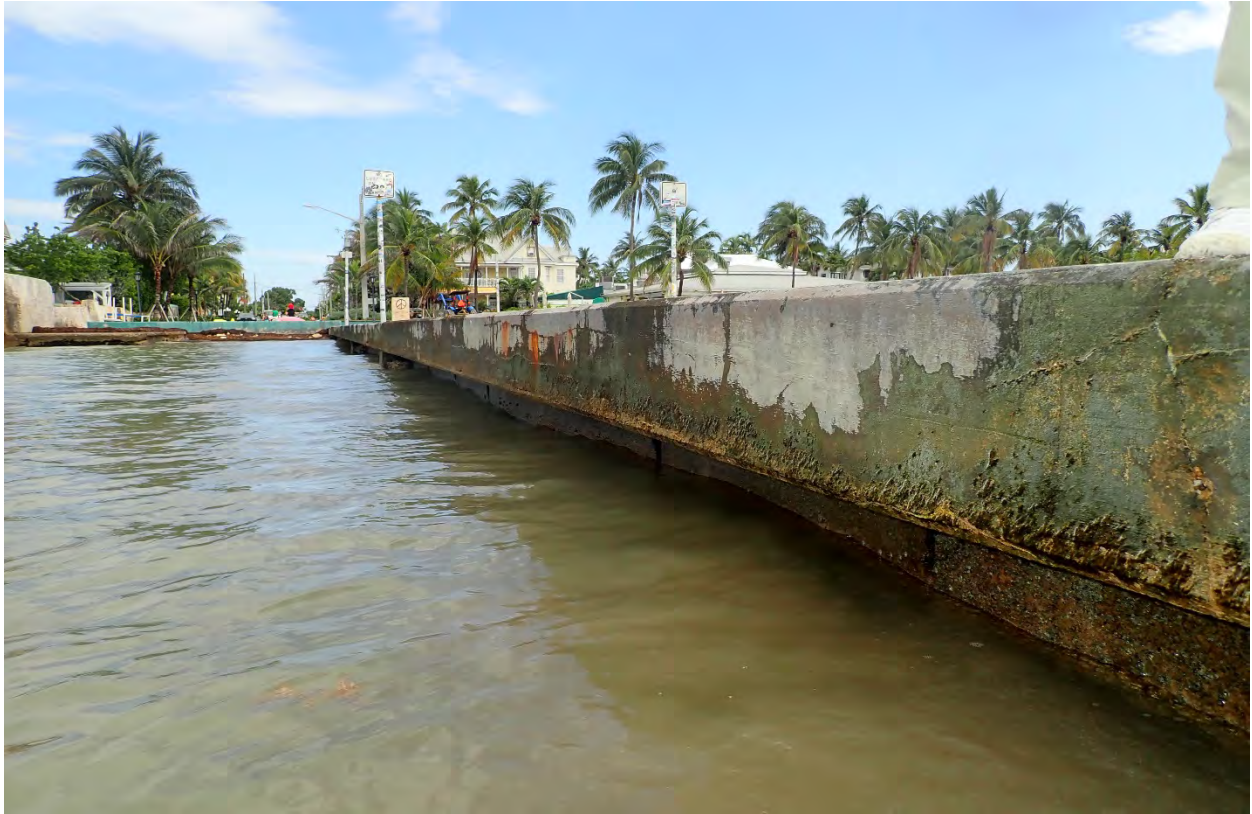
Photo 7. Jetty at the terminus of Duval Street with concrete seawall face. All hard surfaces were inspected for corals.
