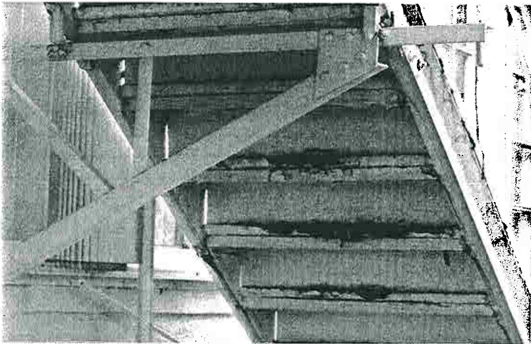
Photograph 17 shows evidence of deferred maintenance at the subject
