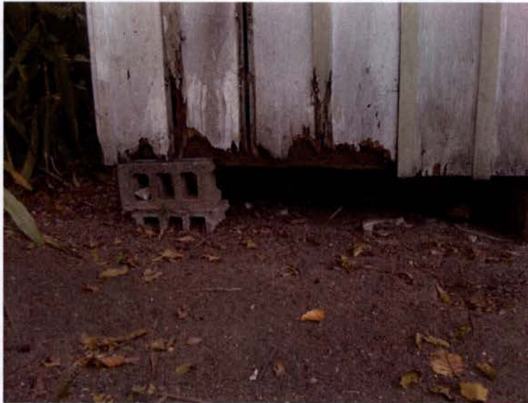
EXISTING BLOCK PIERS TO BE REMOVED AND REPLACED WITH NEW CONCRETE PIERS
