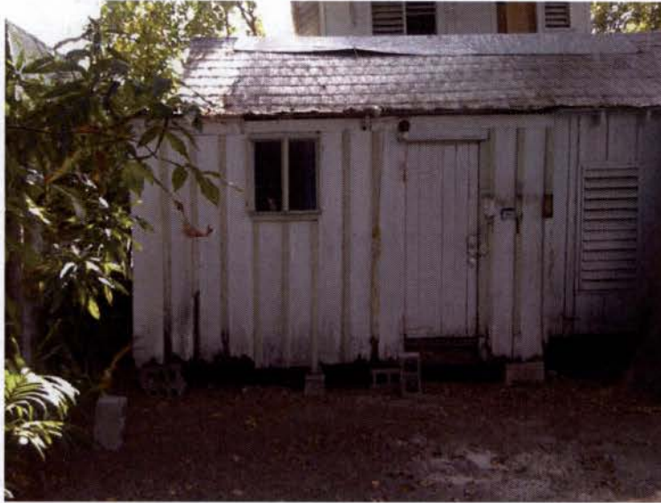
DETERIORATED REAR PORTION OF STRUCTURE TO BE REMOVED AND REPLACED WITH NEW WOOD DECK
