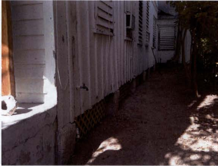
SOUTHEAST SIDE OF THE HOUSE, NEW STAIRS AND COVERED LANDING TO BE INSTALLED HERE
