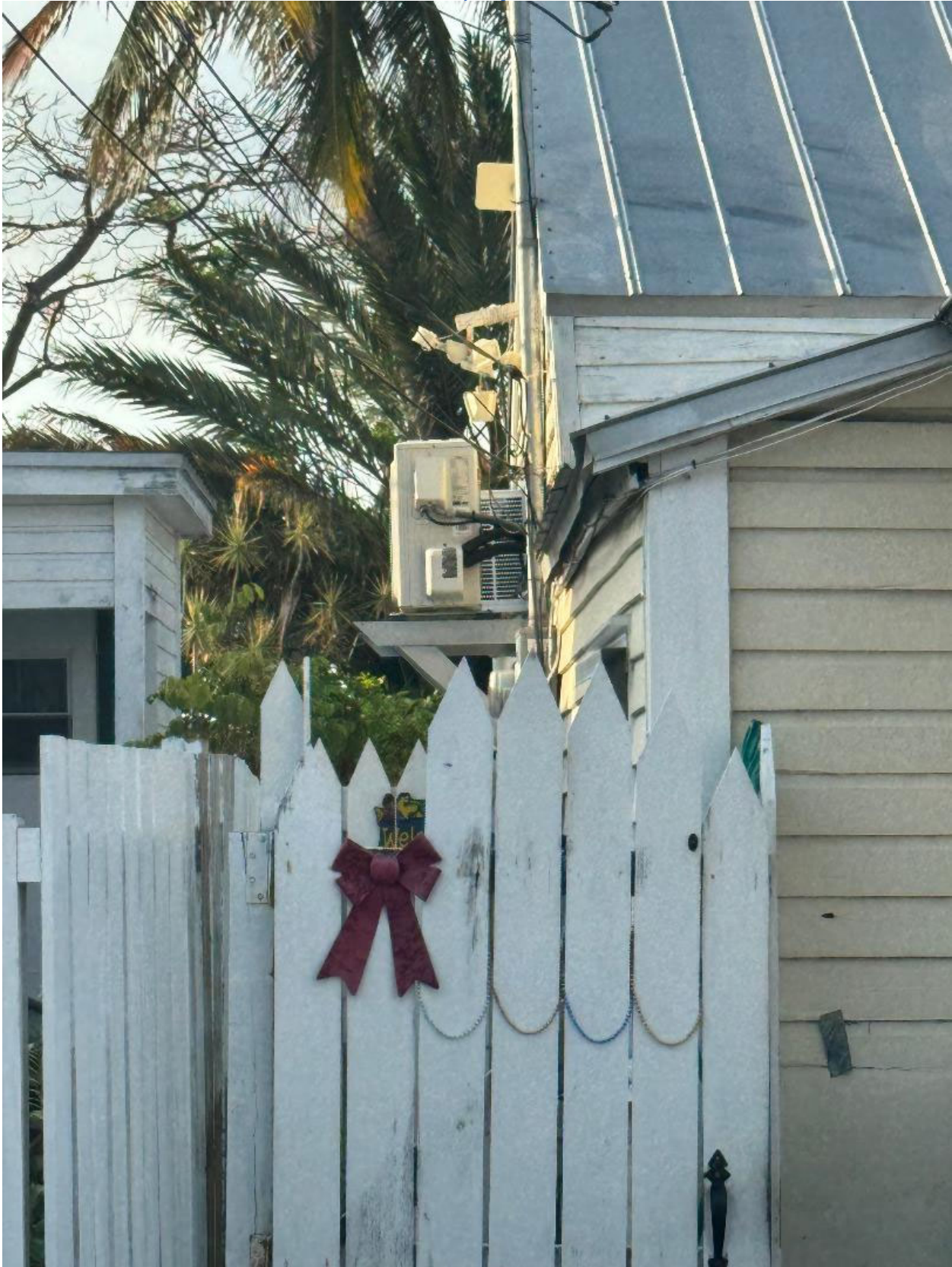
308 Catherine Street – Several Inches from Property line Fence
