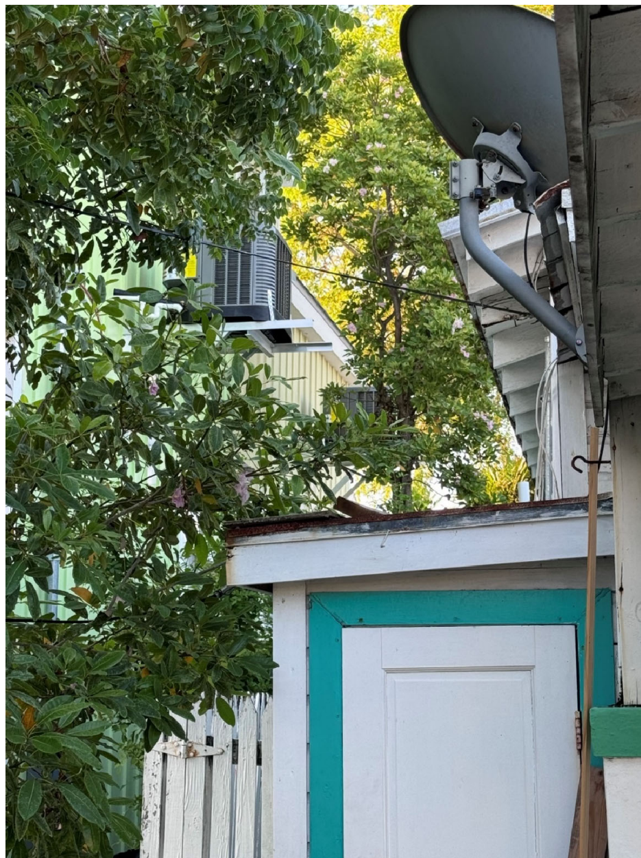
318 Amelia - New Construction , two new AC units installed June 2024
