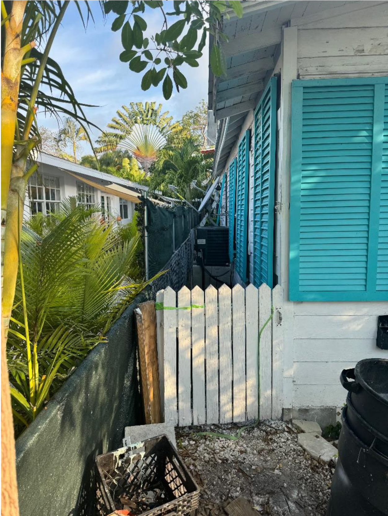
313 Amerlia Street – Inches from Property line fence, poor egress
