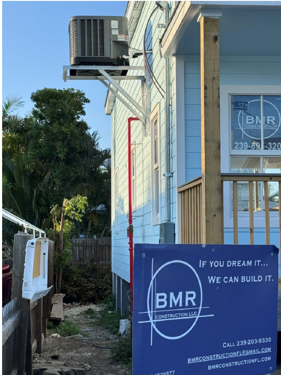
320 Amelia – Coompressor installed wiethin setback June 2024
