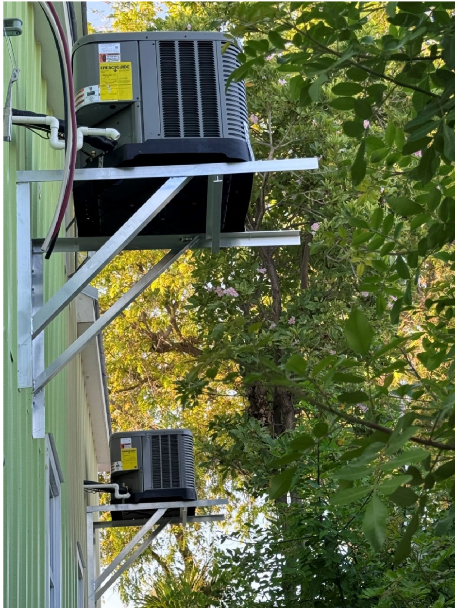
324 Amelia Compressors installed June 2024
