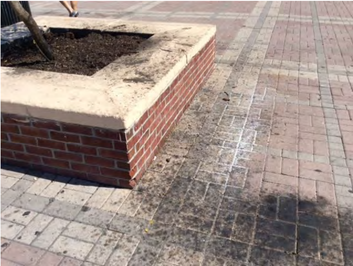
Undated photo showing grease.
