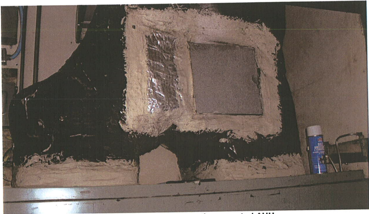
Photo 8: ACM black mastic on central AHU
