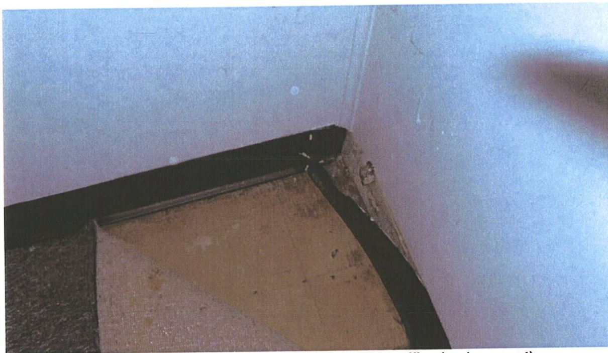
Photo 8: ACM brown VFT/mastic in PIO larger office (under carpet)
