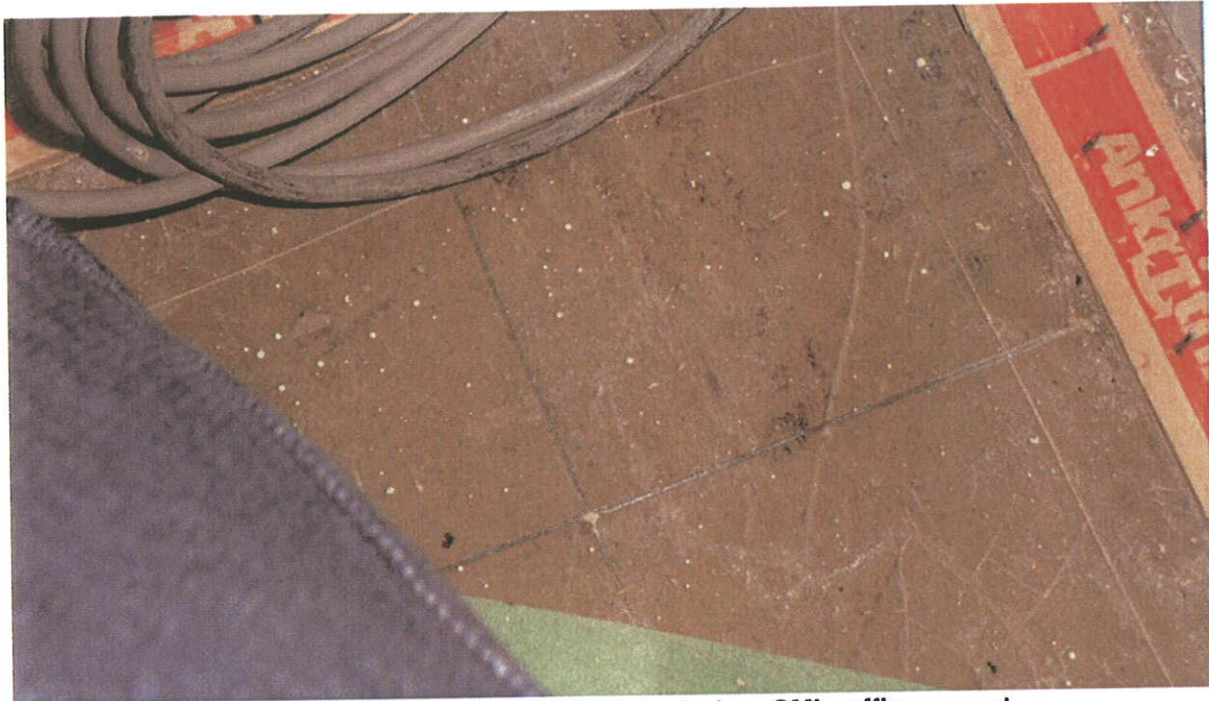
Photo 19: ACM brown VFT/mastic below CM's office carpet
