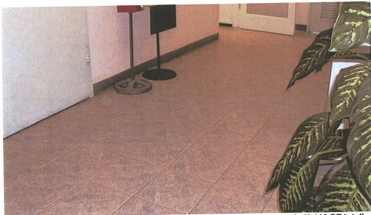
Photo 12: ACM VFT/mastic presumed present beneath floor 2 ceramic (2,110 SF total)
