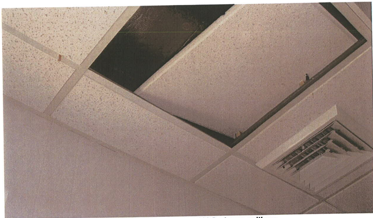
Photo 10: More black HVAC above ceilings
