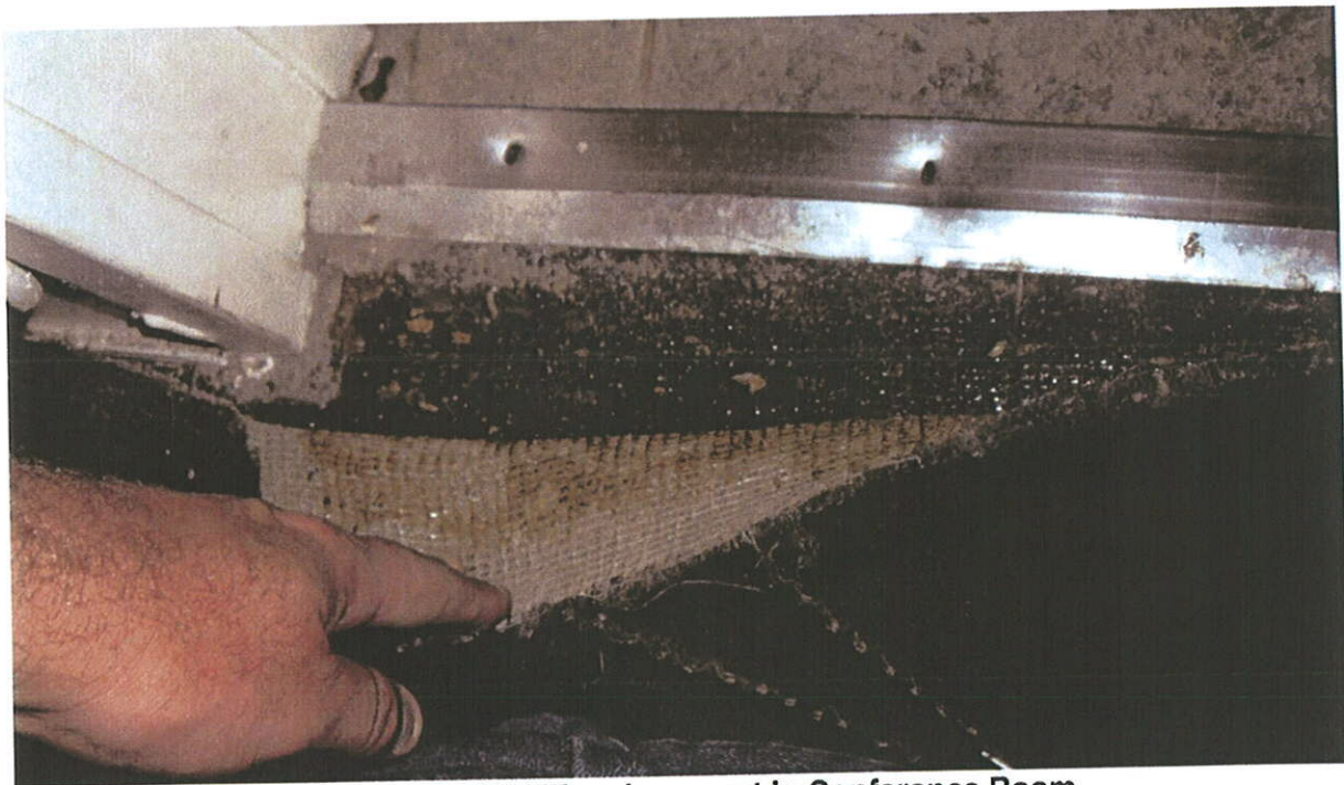
Photo 4: ACM VFT under carpet in Conference Room
