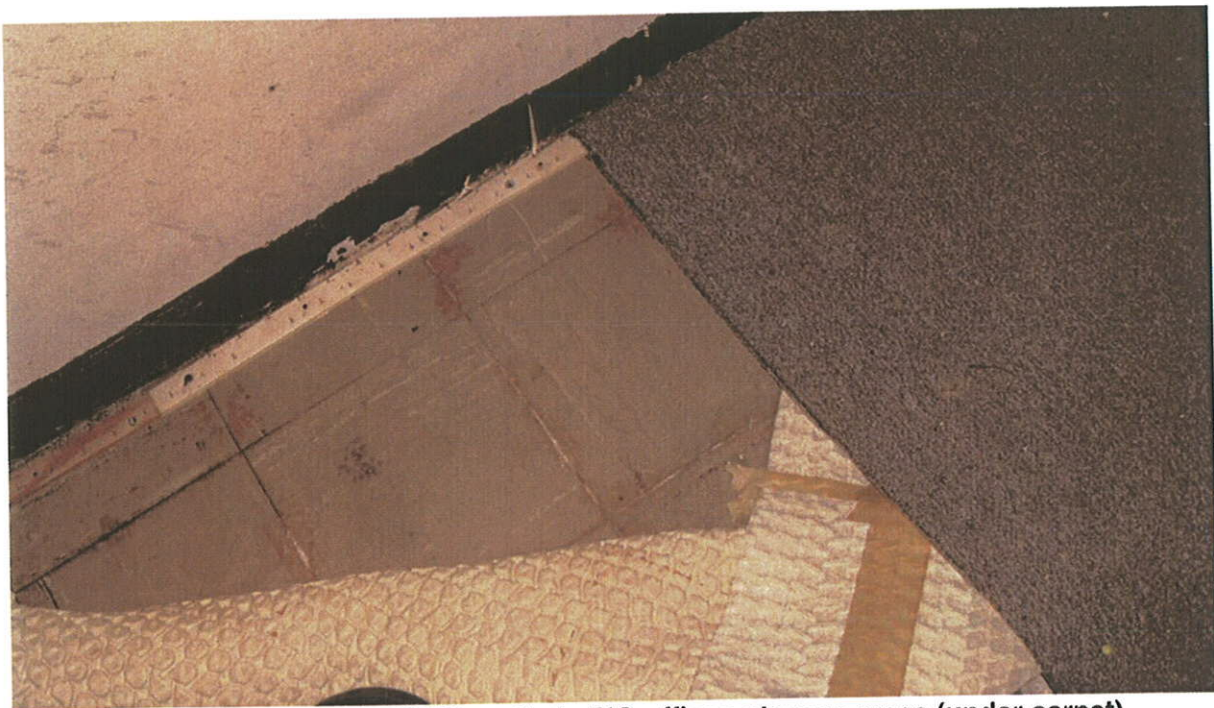
Photo 6: ACM brown VFT/mastic in PIO offices storage areas (under carpet)
