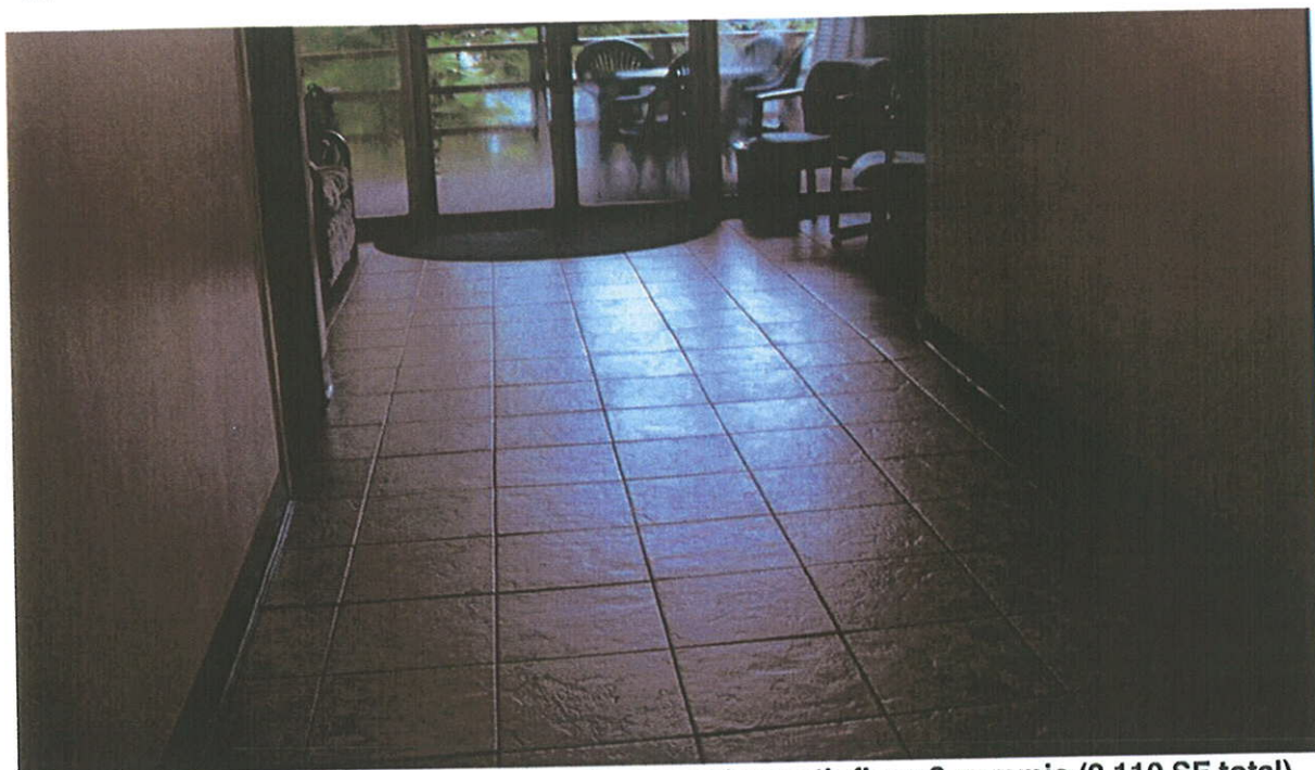
Photo 13: ACM VFT/mastic presumed present beneath floor 2 ceramic (2,110 SF total)
