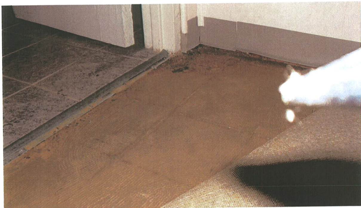
Photo 7: ACM brown VFT/mastic in PIO "LT" office (under carpet)
