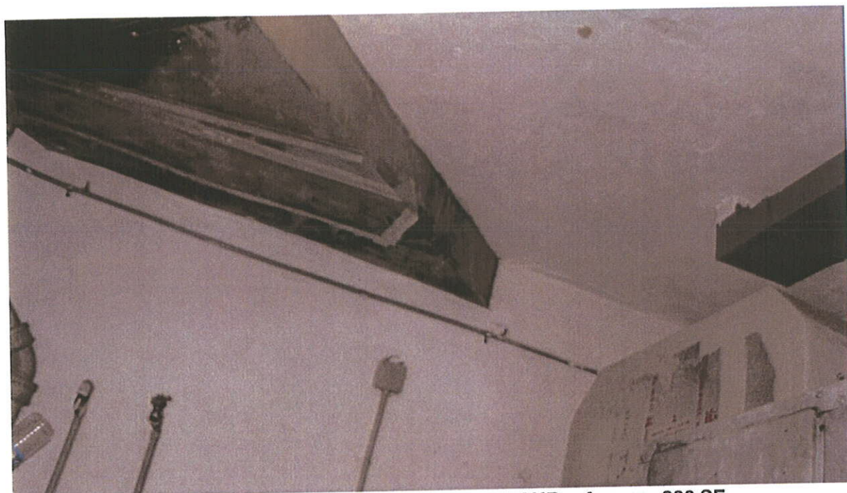
Photo 14: ACM ceiling texture in floor 2 AHR – Approx. 280 SF
