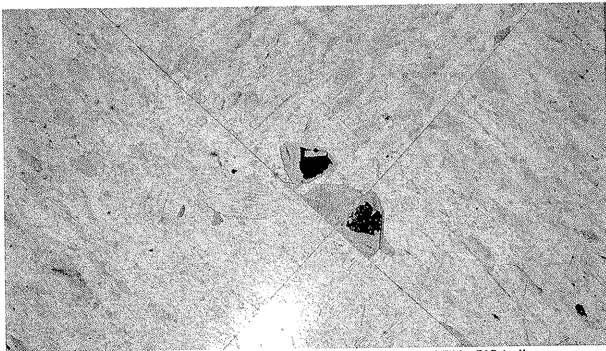
Photo 10: ACM brown VFT/mastic under nonACM VFT in PIO hall
