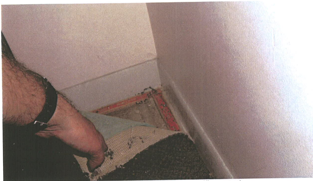
Photo 21: ACM VFT under Portia's office carpet
