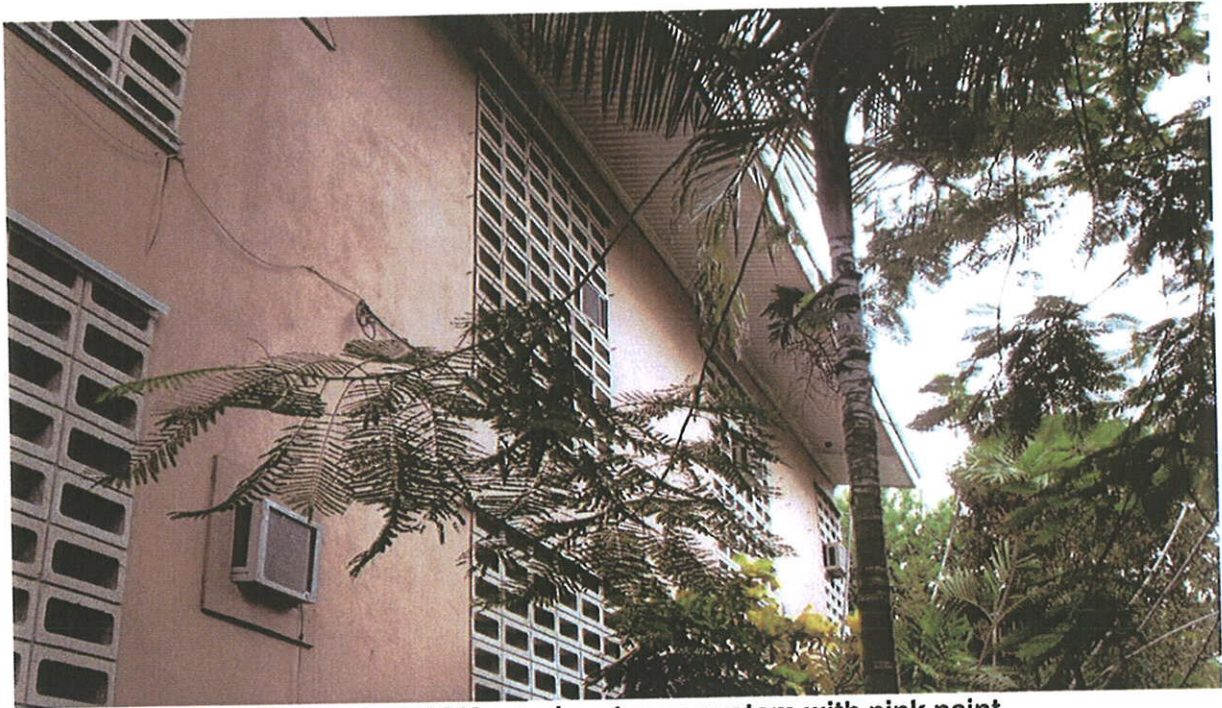
Photo 2: NonACM exterior stucco system with pink paint
