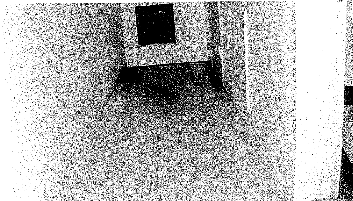
Photo 9: ACM brown VFT/mastic under nonACM VFT in PIO hall
