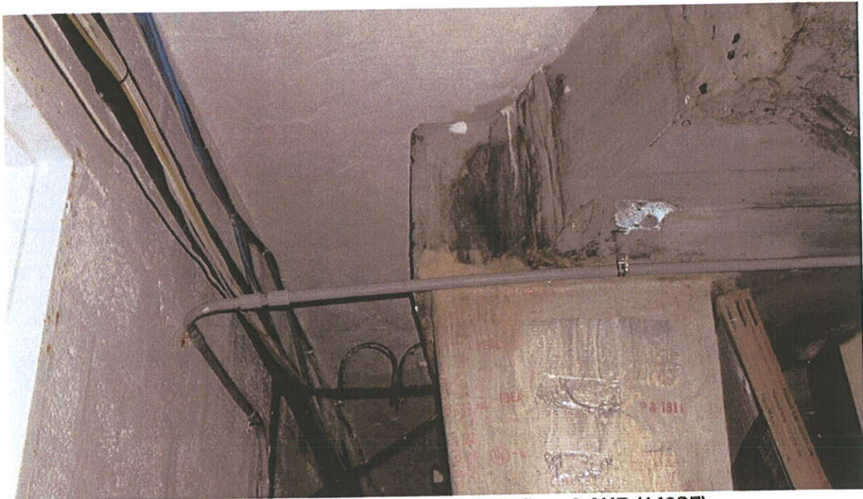
Photo 16: ACM grey HVAC mastic in floor 2 AHR (140SF)
