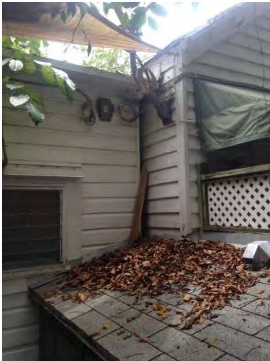
Close up of the connection between the second sawtooth roof and rear gable roof on south side of house. Even though Sanborn maps do not show this as an addition, it looks like one.
