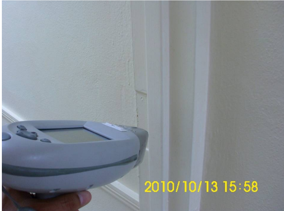
Photograph #4: Interior LBP metal door jamb/casing tested with XRF and sampled for lab analysis during this inspection.
