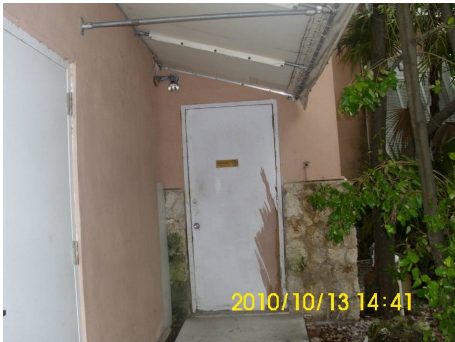
Photograph #2: Typical LBP metal door jamb/casing identified during this inspection.
