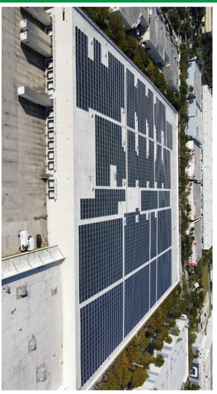
Badia Spices has completed the installation of a rooftop solar array on the company's 300,000-sq-ft distribution and production facility in Sweetwater, Florida. The installation represents the largest
