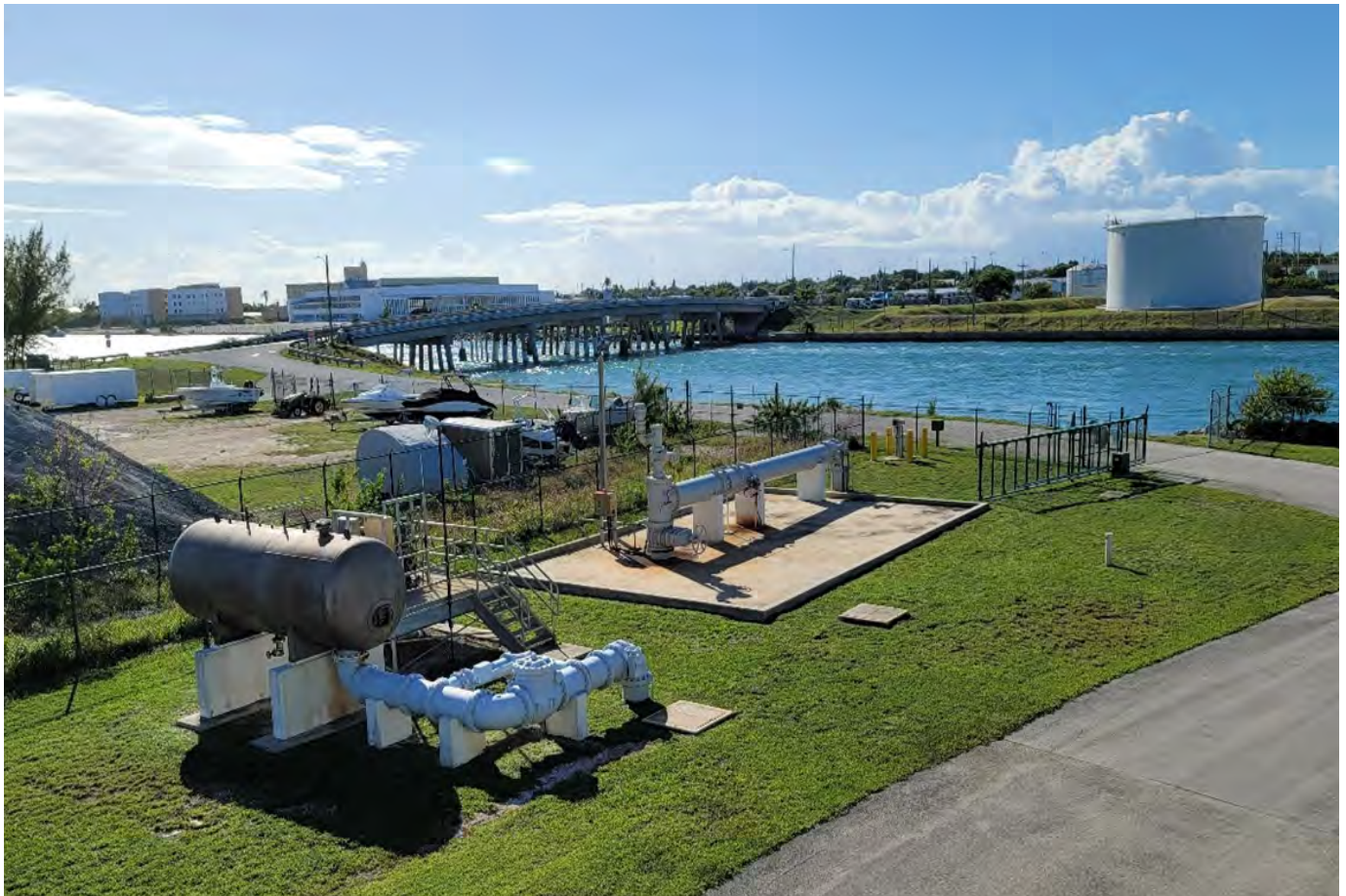
Jacobs has the wastewater treatment plant and injection well expertise and experience to assist the City with fully understanding the risks and stressors on the RAHEPF (photo of surge vessel and deep injection well head at RAHEPF)
