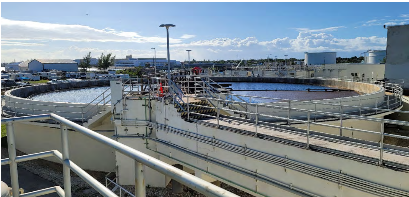
■ Jacobs has the expertise to review RAHEPF treatment processes and recommend resiliency improvements for the plant.
