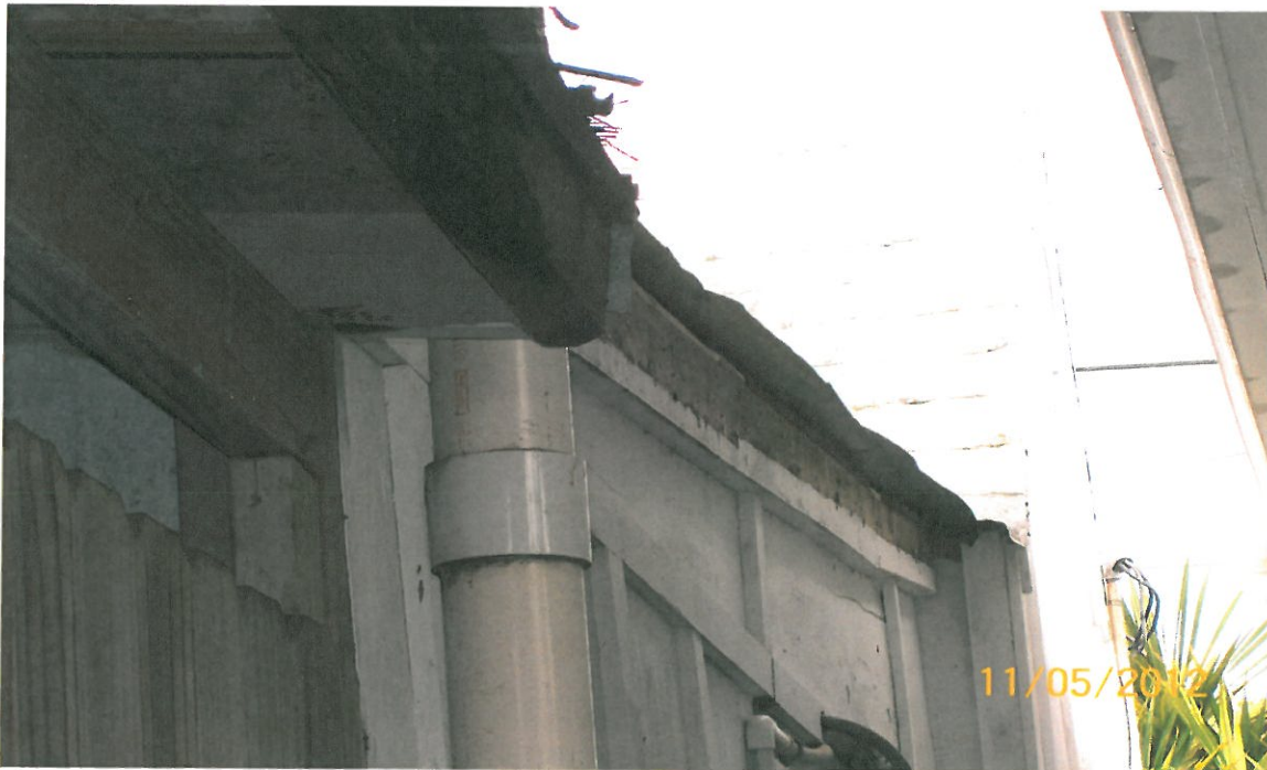
Photo is from neighbor's yard in-between 1010 on left and 1012 on right. New wood supports and what appeared to be a "Hurricane clamp" (center of photo) were visible on right side of roof.
