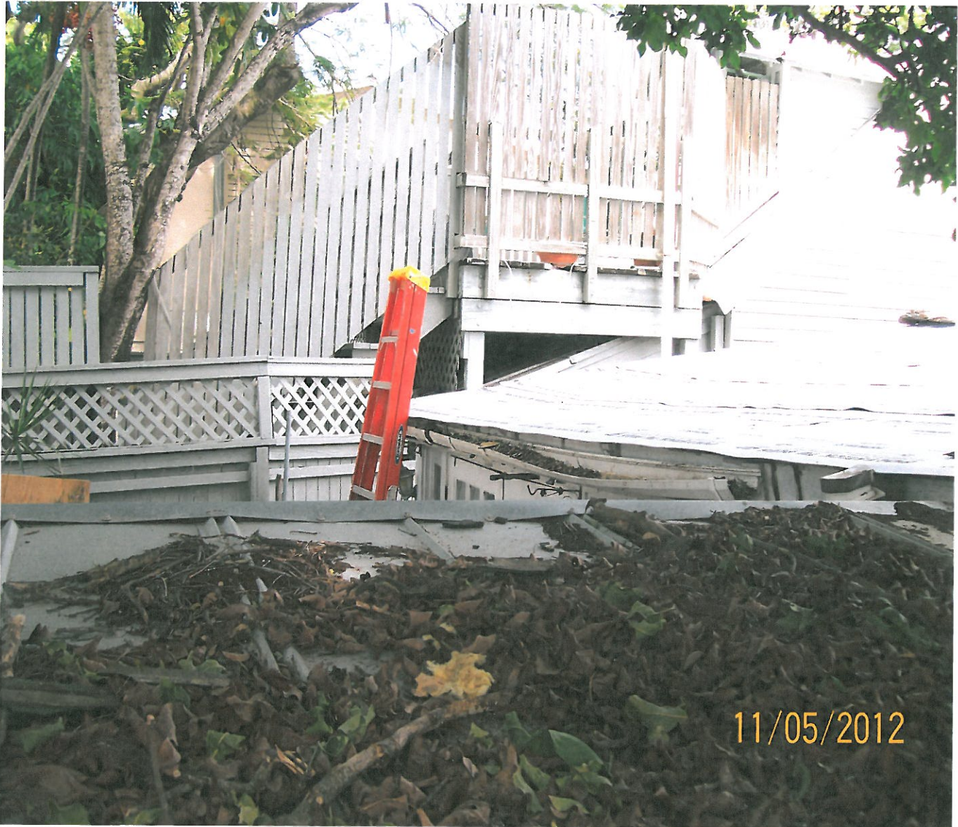
This photo is from neighbor's yard, looking above shed at 1010 Whitehead St.
