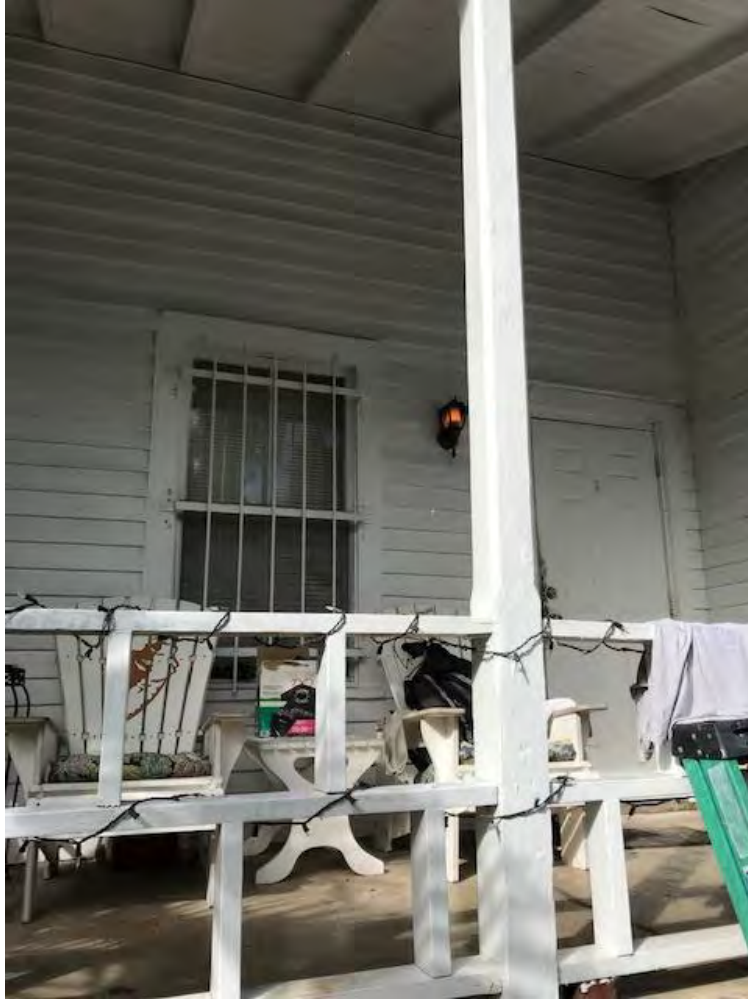
Partial view of east elevation showing historic window and non-historic door to be replaced with sliders.
