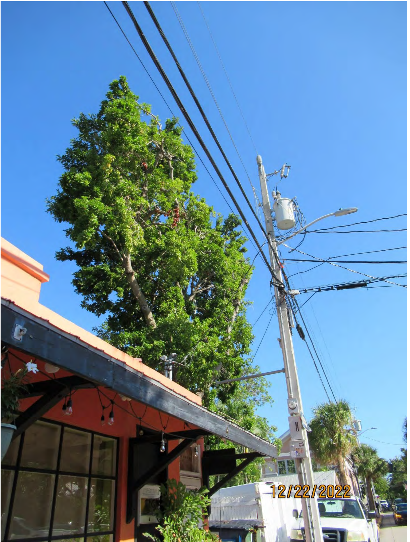
Photo of tree and its canopy in relation to the utility lines.
