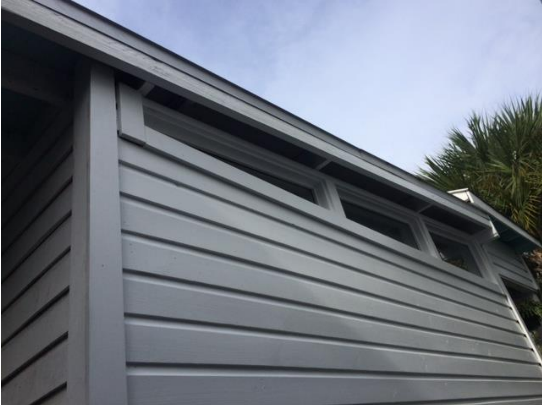
Close-up of side addition. The side wall and window will remain. A new gable roof will be constructed on top.
