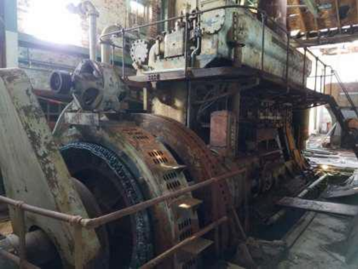
Dynamo generator in Building 1, Unknown manufacturer, Diesel Plant structures, Key West, Florida. Source: Enid Torregrosa, Historic Preservation Planner
