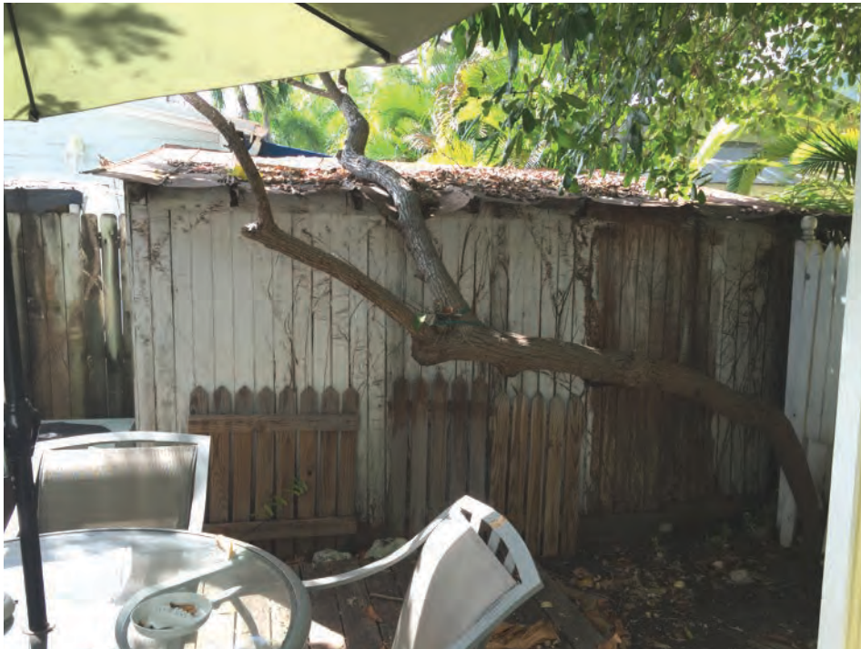
Back side of shed to be demoed, encroaching on neighbor's property to the north
