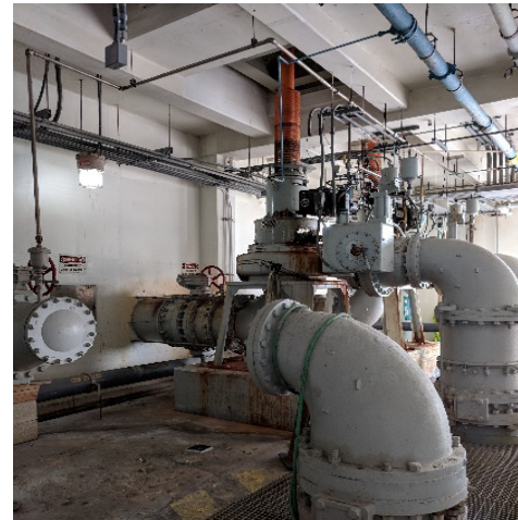
Figure 4-6. Deep Well Pumps with Future Pump Location
