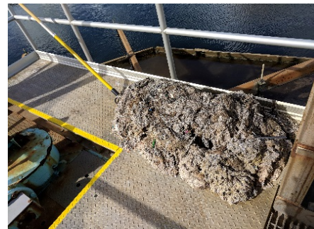
Figure 4-8. Rags Collected from Secondary Clarifier
