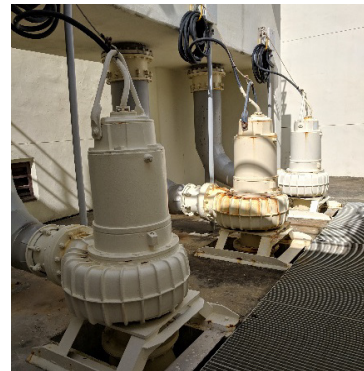
Figure 4-11. Filter Influent Pumps
