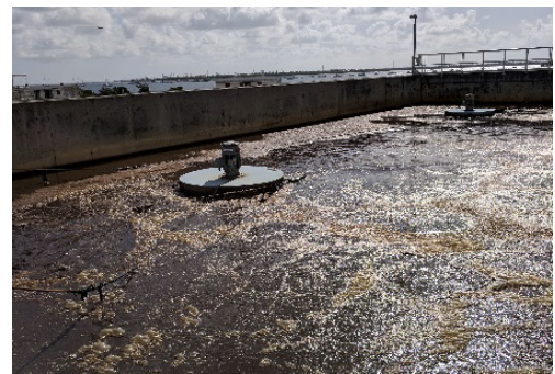
Figure 4-7. Scum Trapped from the Aerobic to Pre-anoxic Zone Backflow Induced by Airlift
