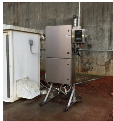
Figure 4-12. ZAPs Liquid Station for UV Dose Control
