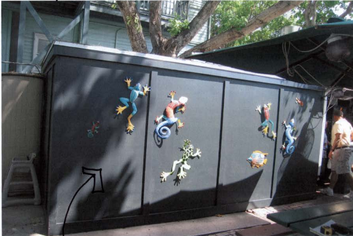
EXISTING PLYWOOD ADDITION TO NEAR OF EXISTING KITCHEN BUILDING TO BE REMOVED
