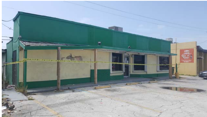
Image of the existing, damaged structure, with yellow “caution” tape wrapped around it.
