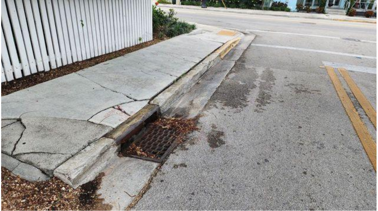
Photo 6 (Damage to the sidewalk and drain area on Packer Street)
