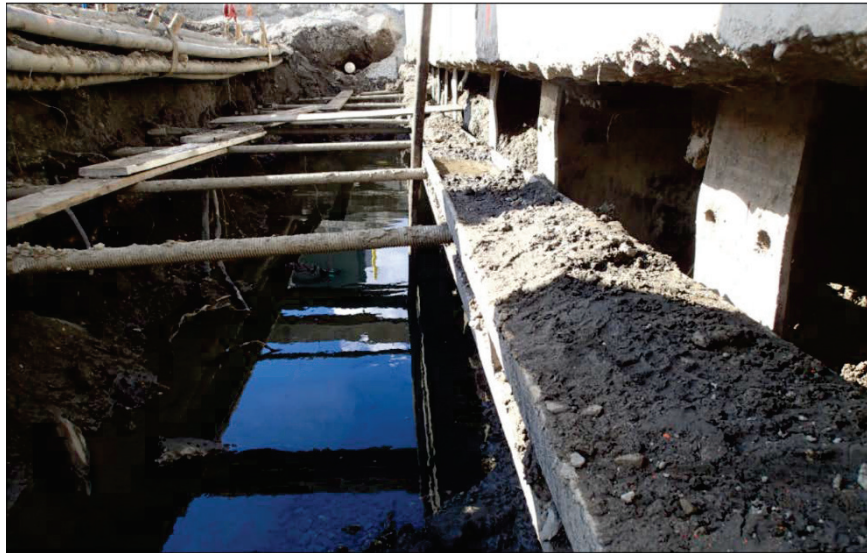
Colonna's Shipyard bulkhead failure
