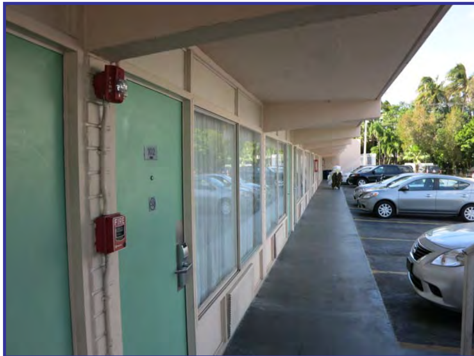
View looking west along the north elevation of building A - ground floor
