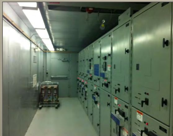
Inside the control building
