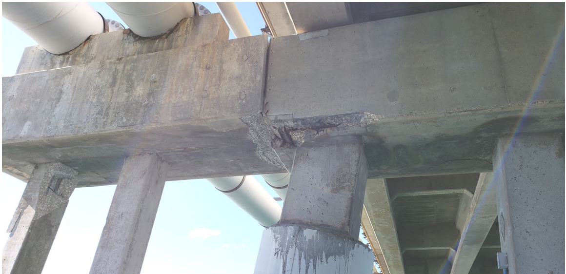
Figure 1. Top bent of the utility bridge supporting two 32" sanitary influent lines and results of an impact of the bent into Navy owned vehicular bridge.
