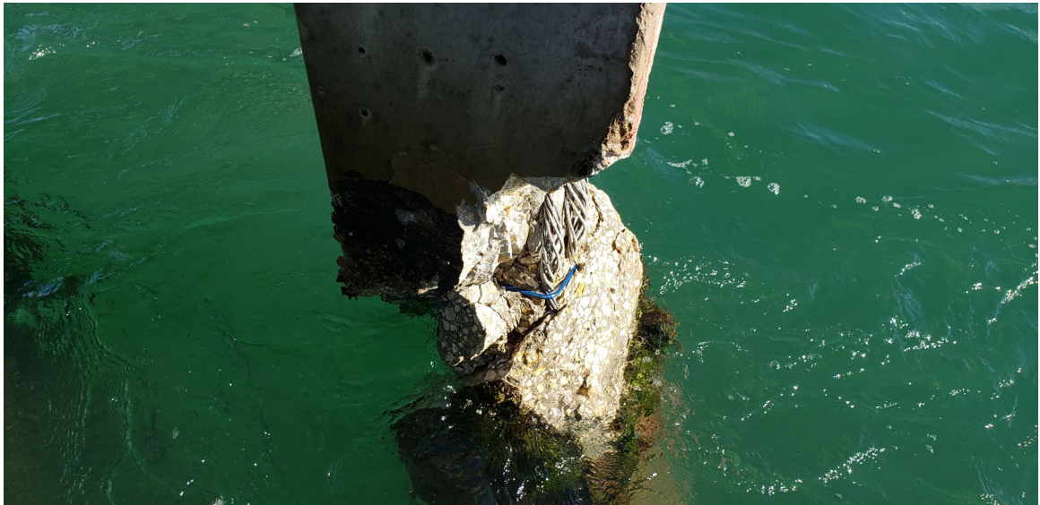
Figure 4. Outer pier at water level. Complete loss of section and damage to reinforcement tendons.
