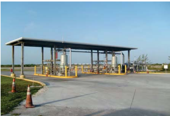
Jet Fuel Pump Station, Boca Chica NAS
