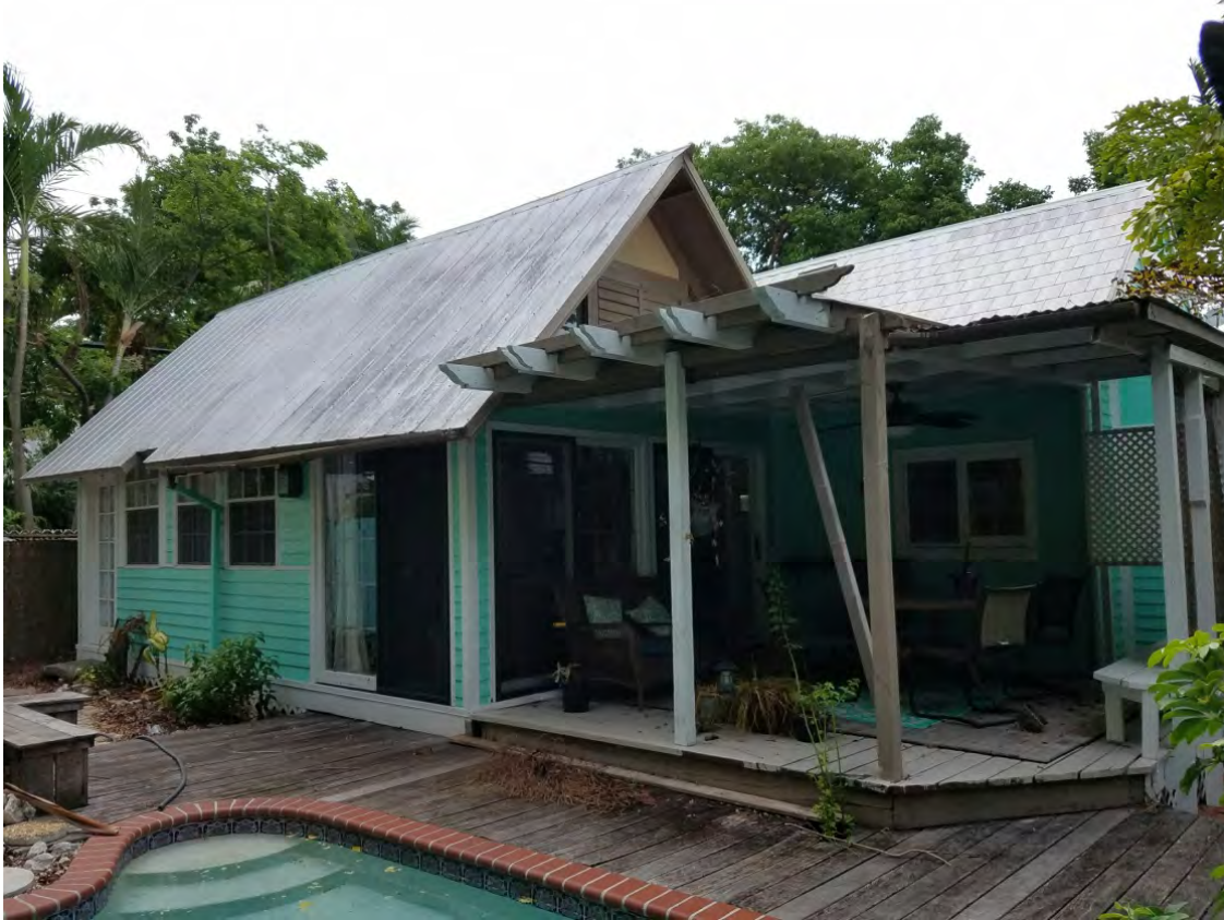
Side (west) façade. Note: this addition was constructed after 1968. Replace all doors and windows with painted wood units. New bifold doors. Repair existing porch roof. New wood decking.
