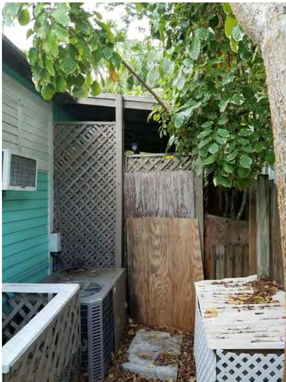
Side (east) façade. Remove and replace all aluminum doors and windows. Cut back existing overhang to comply with setbacks.
