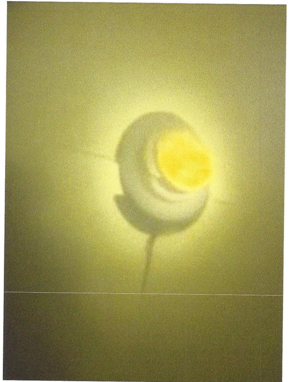
(Photograph showing damage to CP jacket around pumping port)
