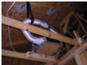
Poor installation (U bend)
