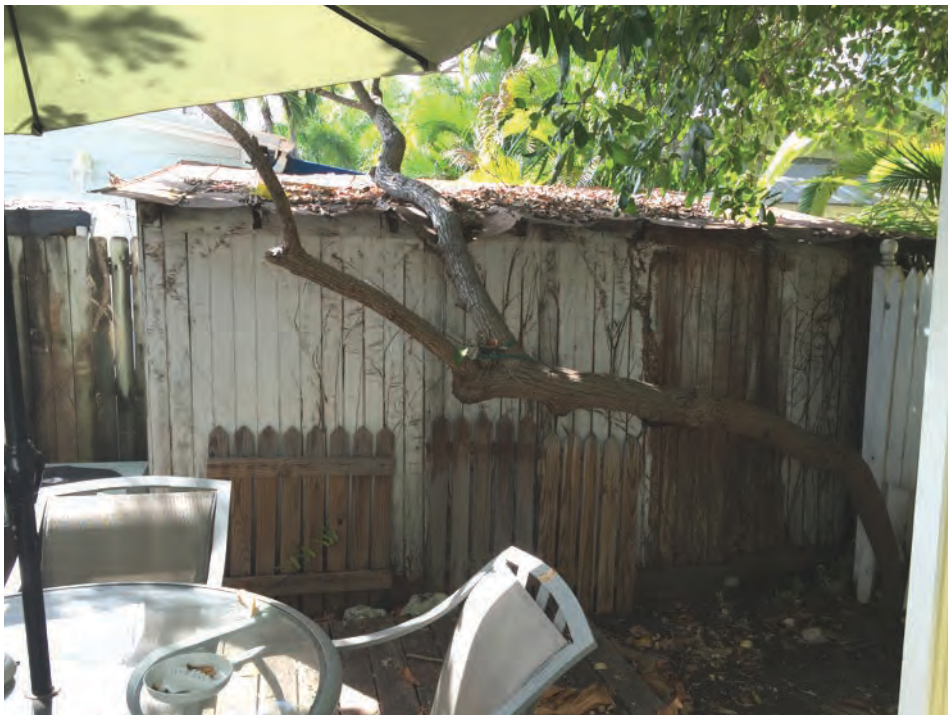
Back side of shed to be demoed, encroaching on neighbor's property to the north
